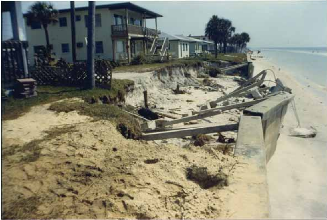
FIGURE 74. Elena damaged 23rd Avenue
