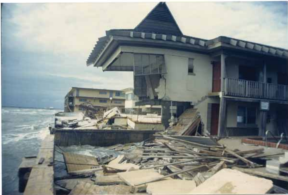
FIGURE 122. The Islander after Juan's additional damage
