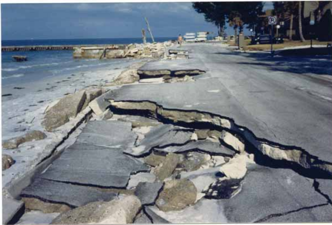
FIGURE 151. Beach Road damaged on Siesta Key (S. West)
