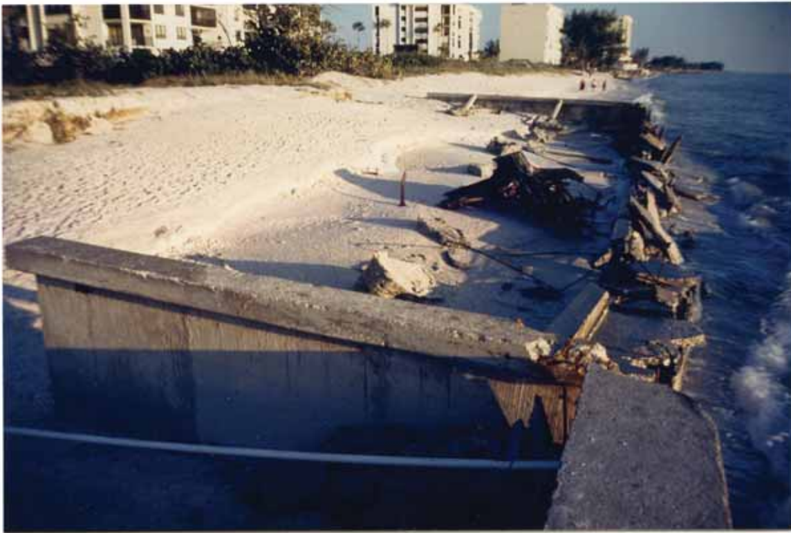
FIGURE 147. Juan destroyed concrete bulkhead
