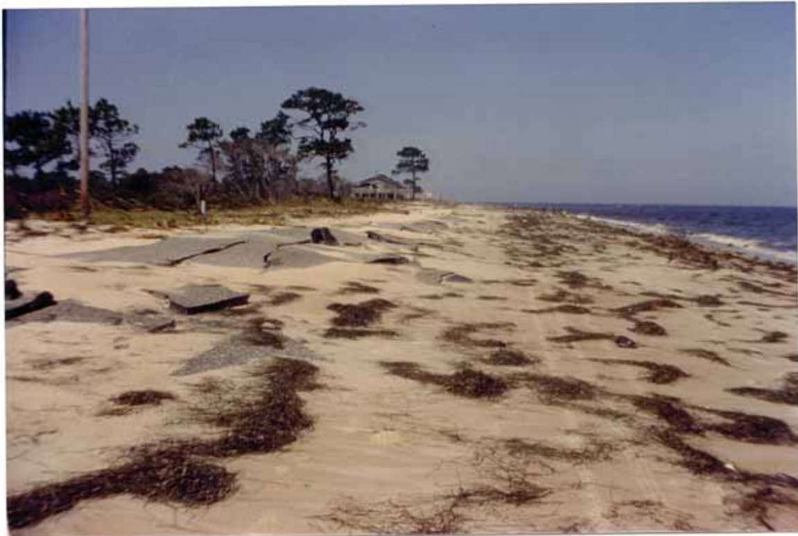
FIGURE 45. Lighthouse Point road destroyed on September 1
