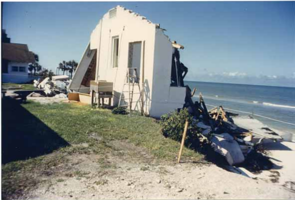
FIGURE 81. Dwellings destroyed at 17th Avenue
