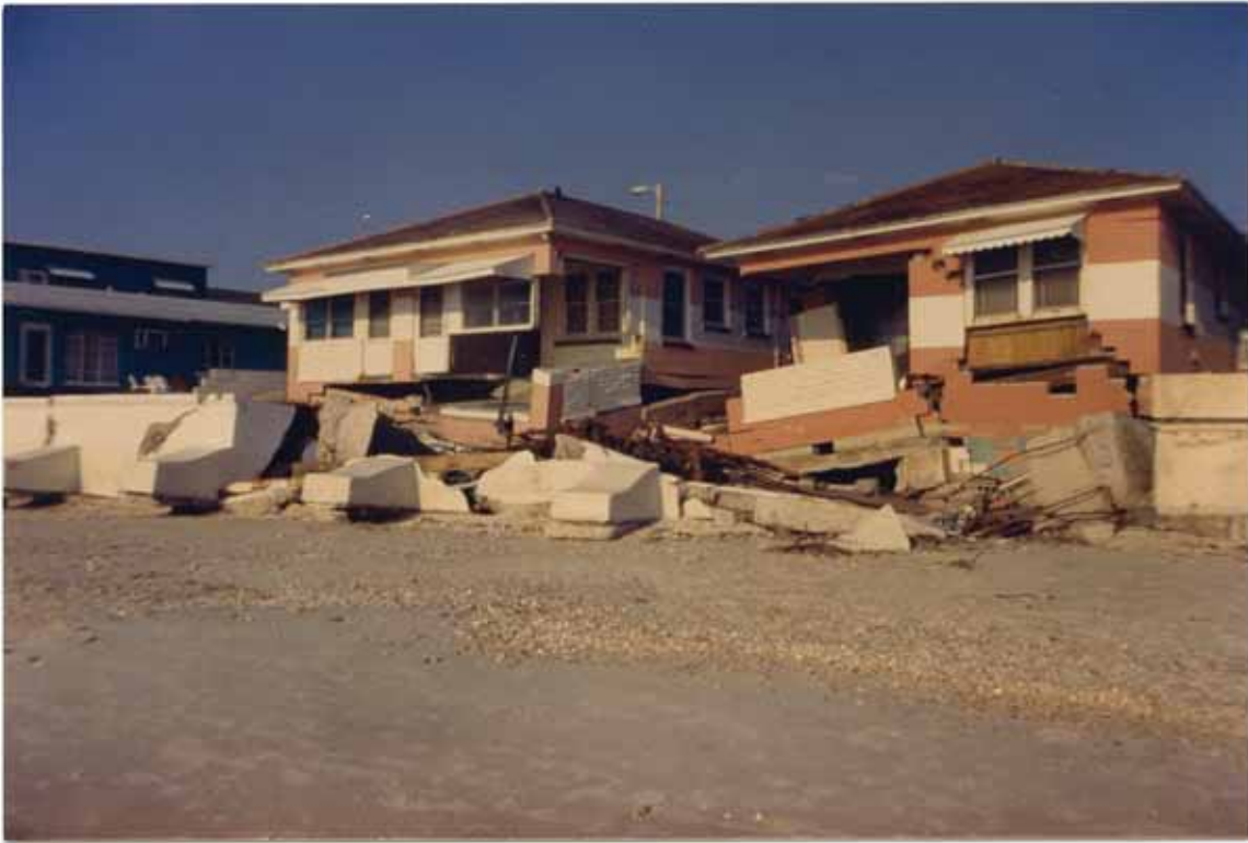
FIGURE 107. Wall destroyed and dwellings damaged
