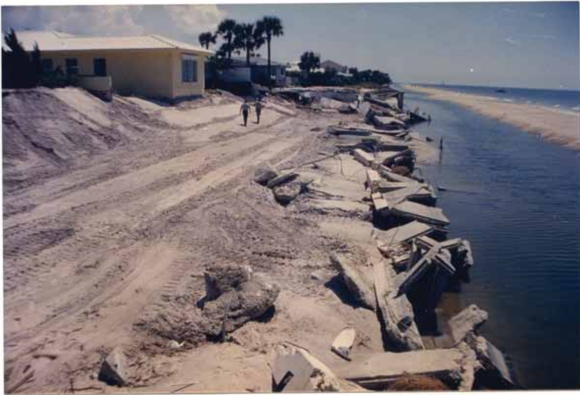
FIGURE 64. Concrete bulkhead destroyed, 650 feet
