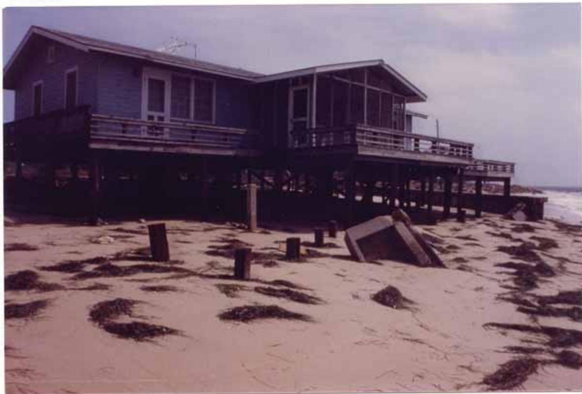
FIGURE 29. Southwest Cape bulkhead destroyed by Elena's waves
