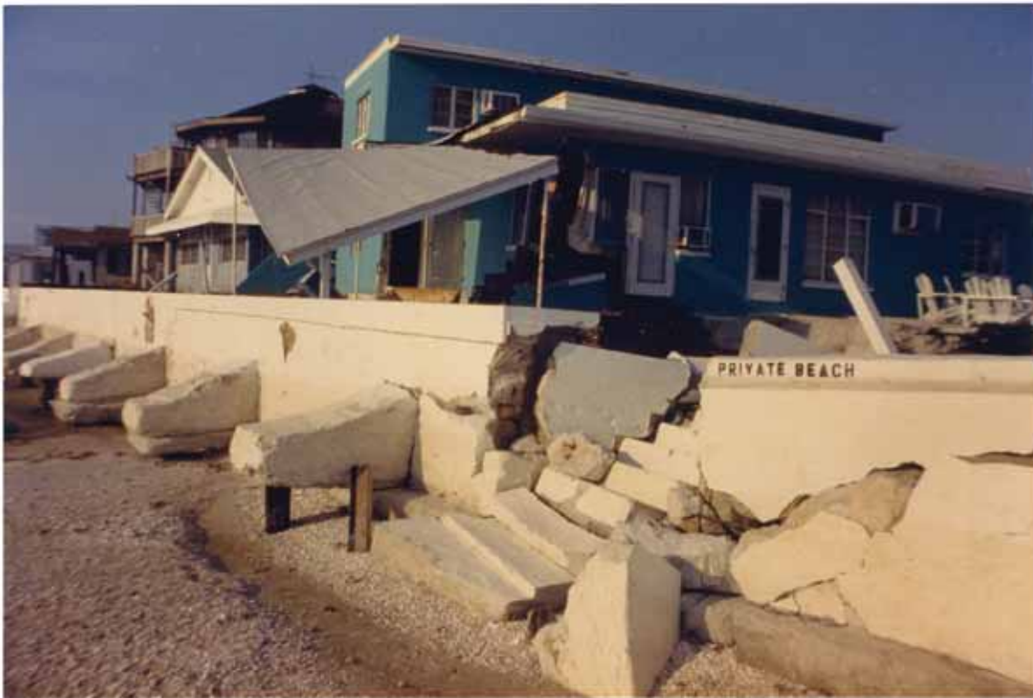
FIGURE 106. Wall damaged by wave impact loads
