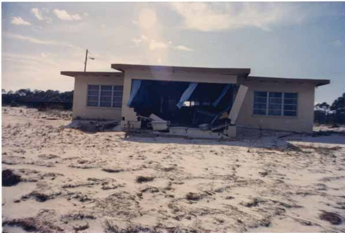
FIGURE 43. Elena's waves damaged dwelling near Bald Point
