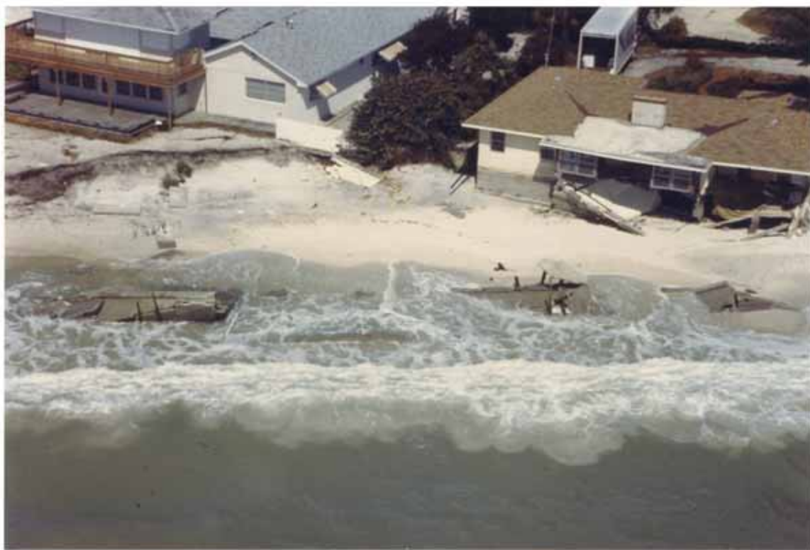
FIGURE 128. Dwelling damaged by Elena
