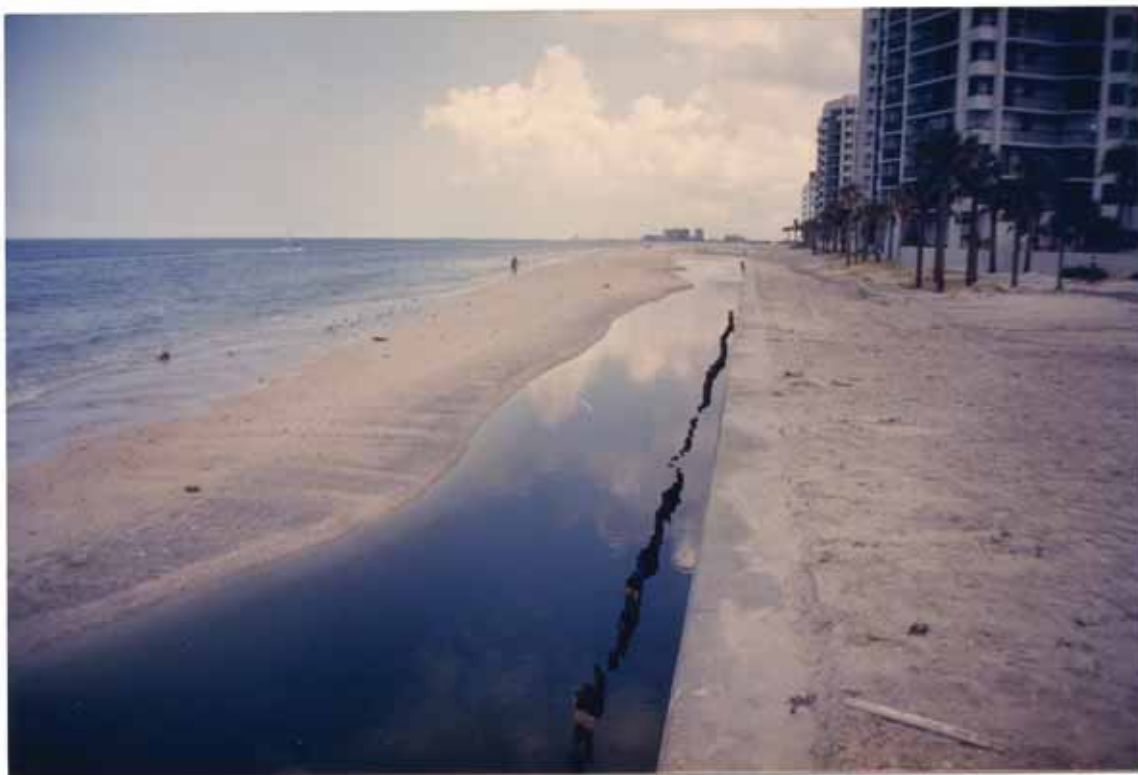
FIGURE 51. Scoured beach adjacent vertical bulkhead
