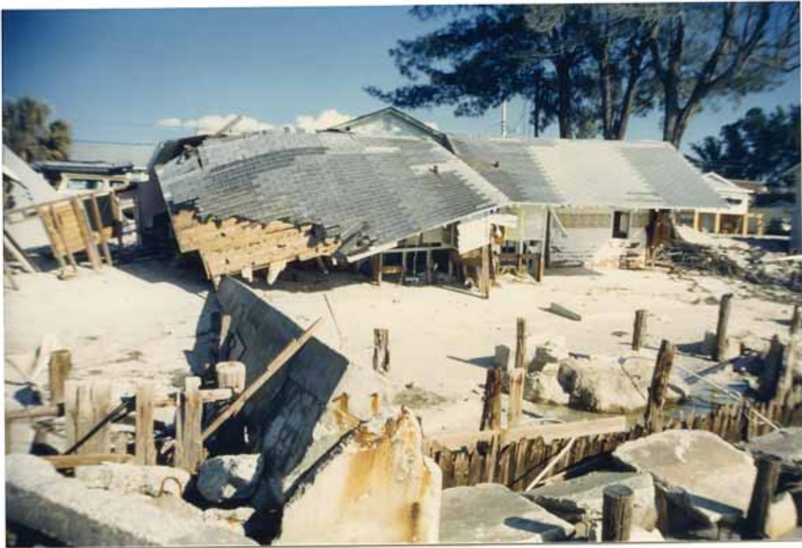
FIGURE 136. Bradenton Beach dwelling destroyed by Elena
