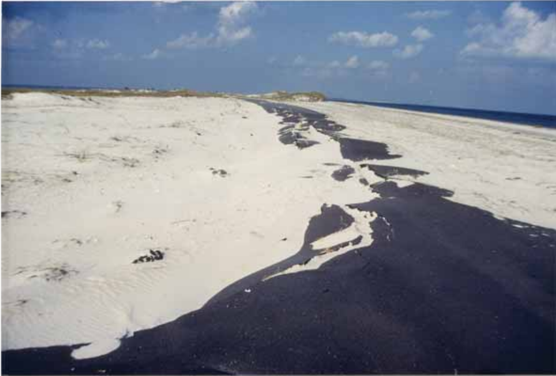
FIGURE 10. Park road segment destroyed by Elena, St. George Island
