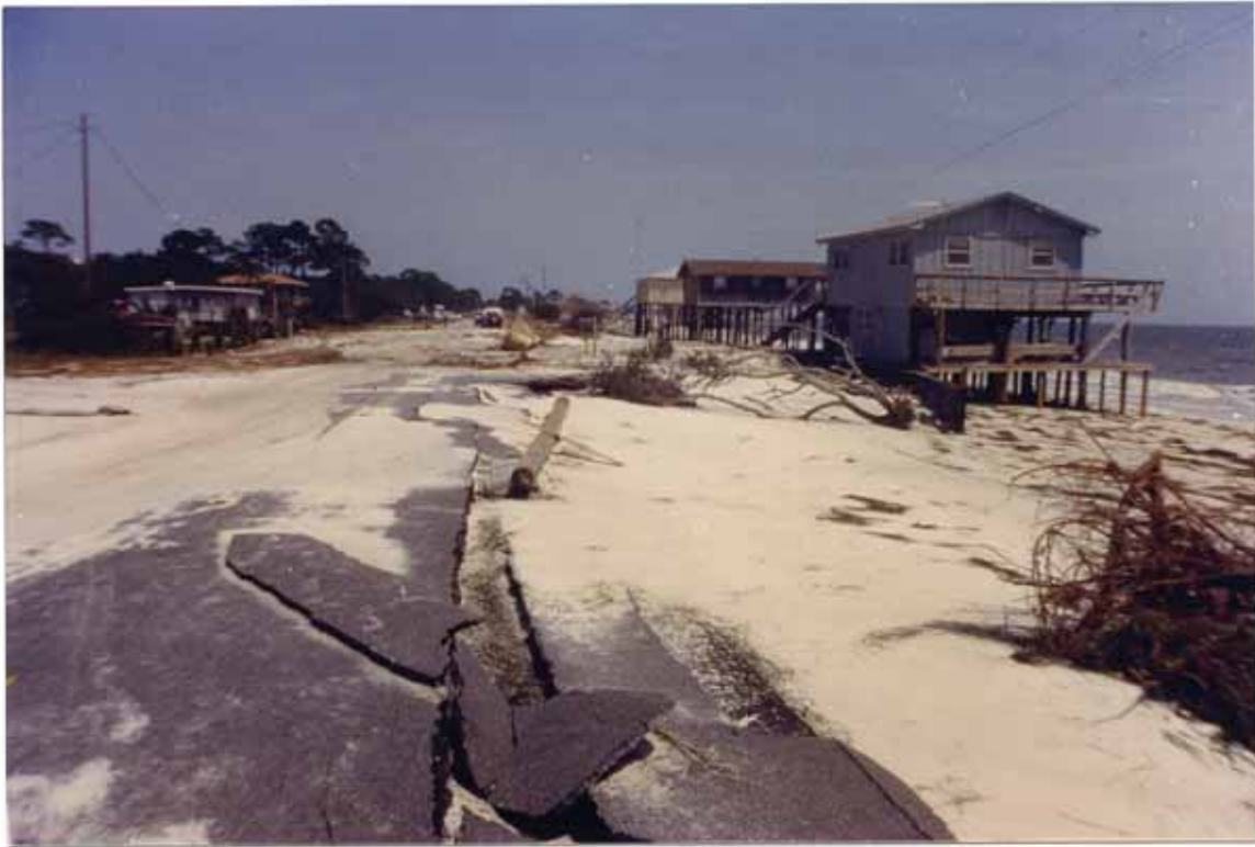
FIGURE 32. Elena erosion and damage
