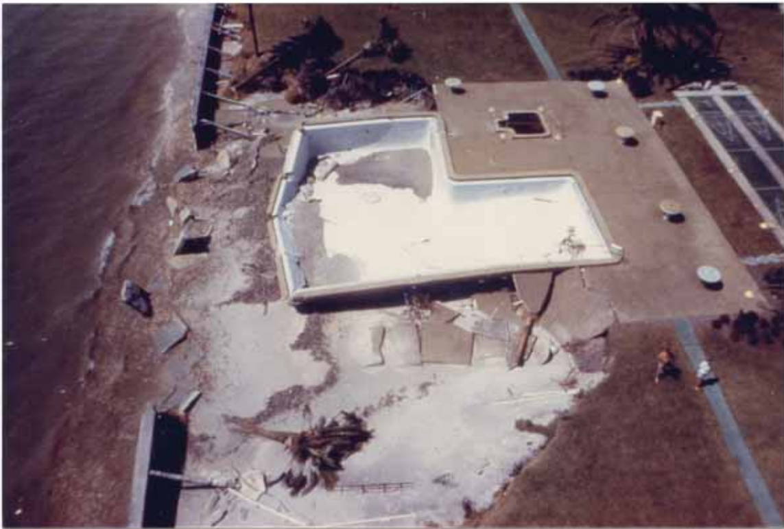
FIGURE 115. Wall and pool destroyed, Shore Mariner Condominium
