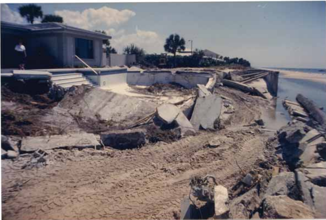
FIGURE 65. Wall and pool destroyed
