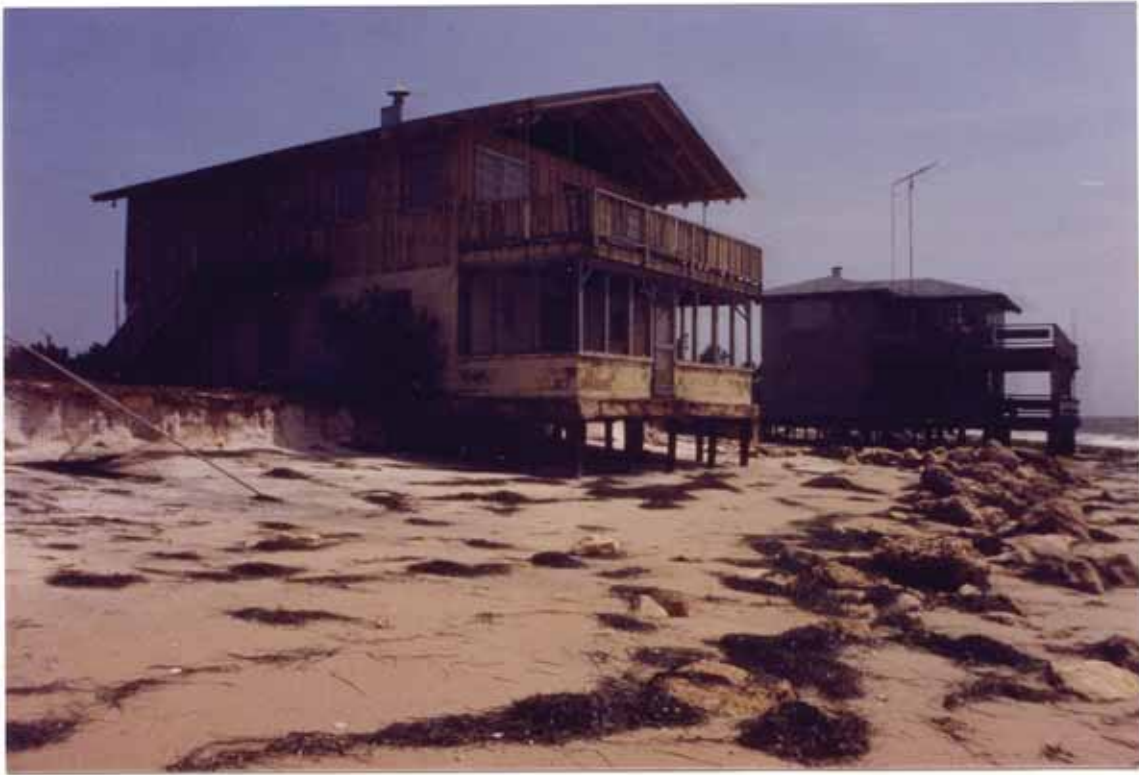
FIGURE 28. Southwest Cape revetment destroyed and dwelling undermined
