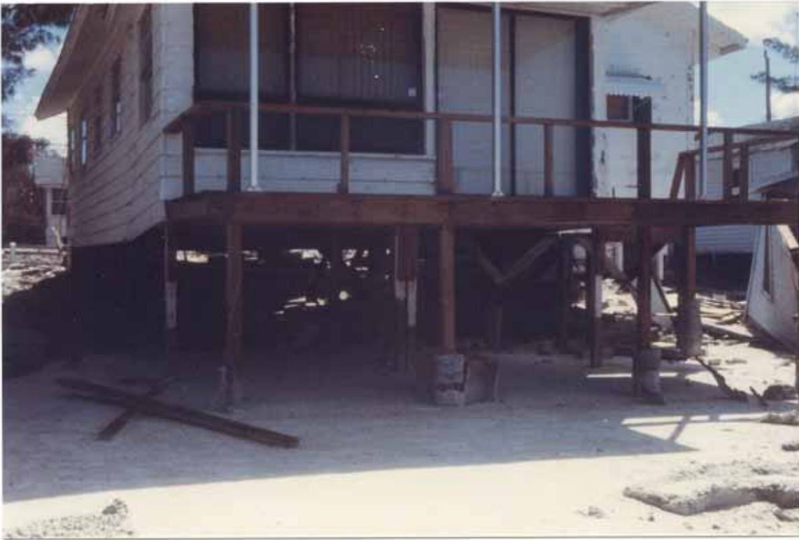
FIGURE 137. Bradenton Beach dwelling damaged by Elena (S. West)
