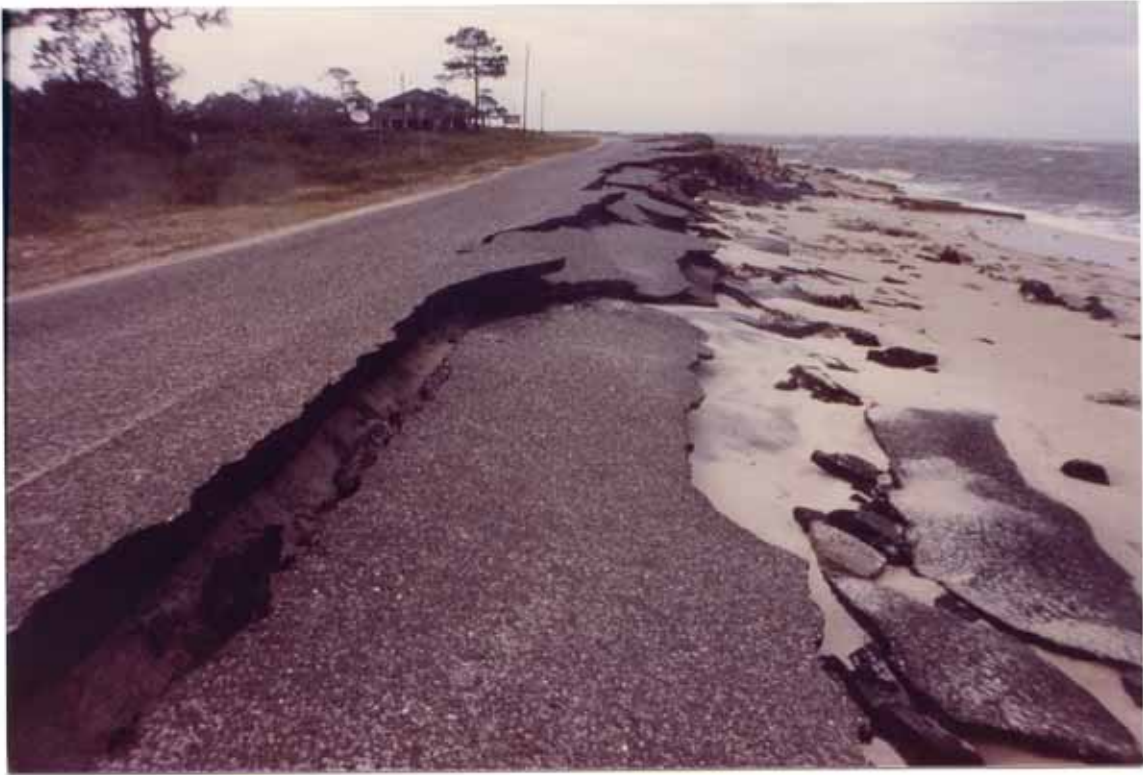
FIGURE 46. Lighthouse Point road damaged on August 30
