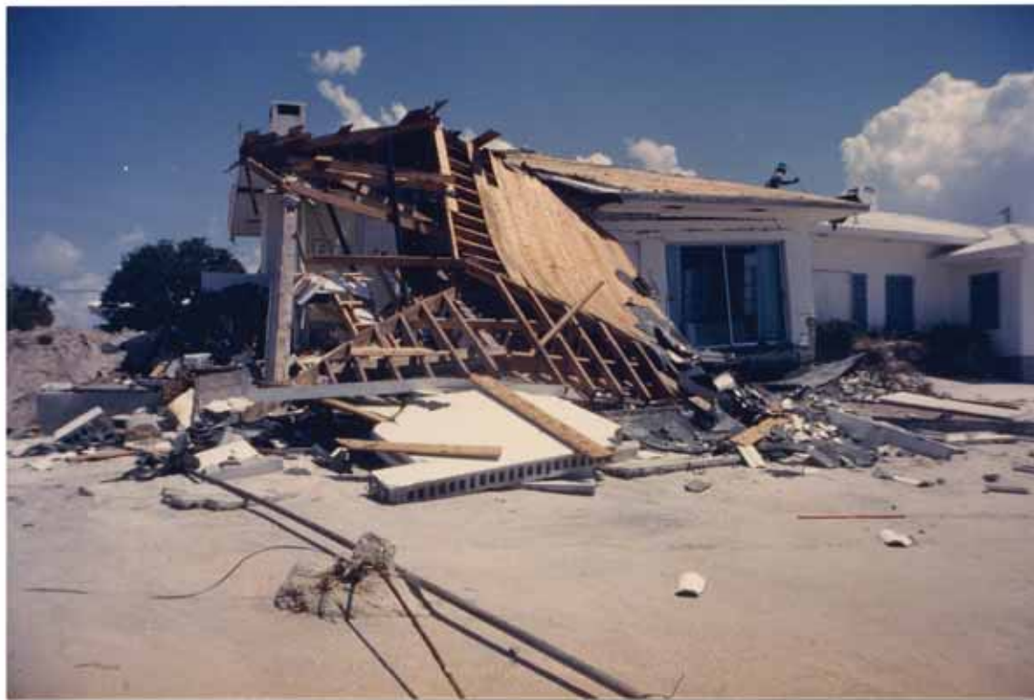
FIGURE 63. Belleair Shore dwelling damaged
