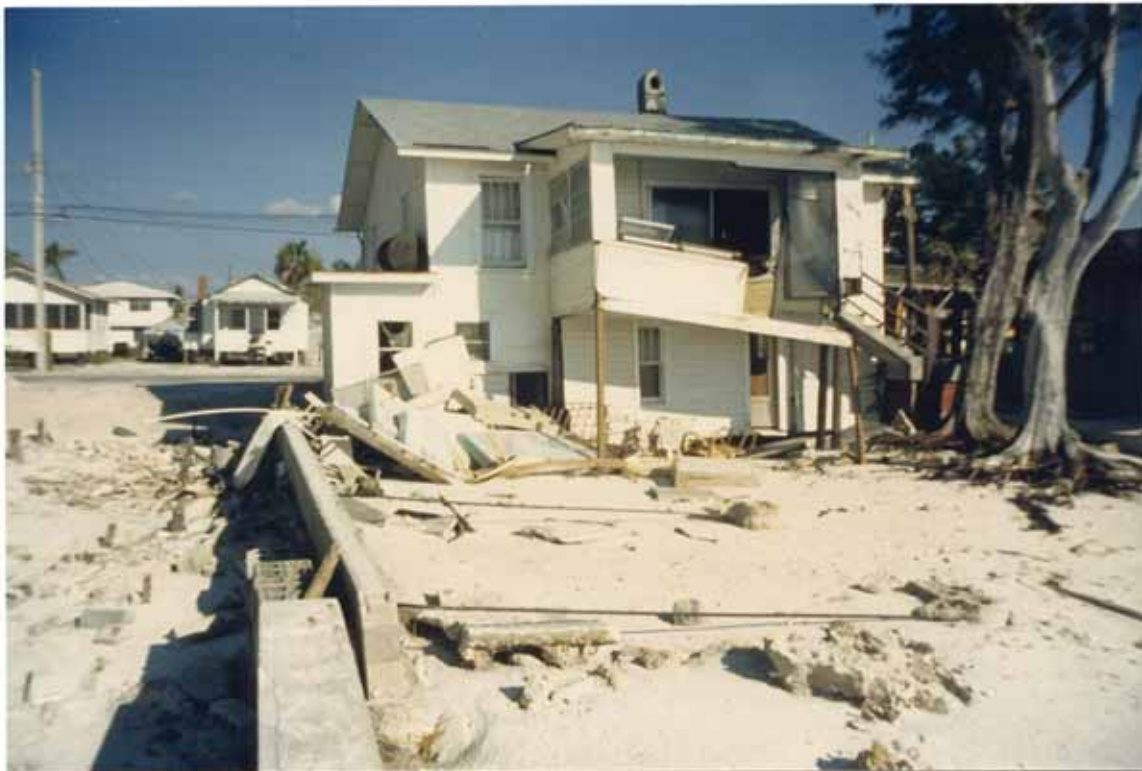
FIGURE 140. Dwelling damaged and settled
