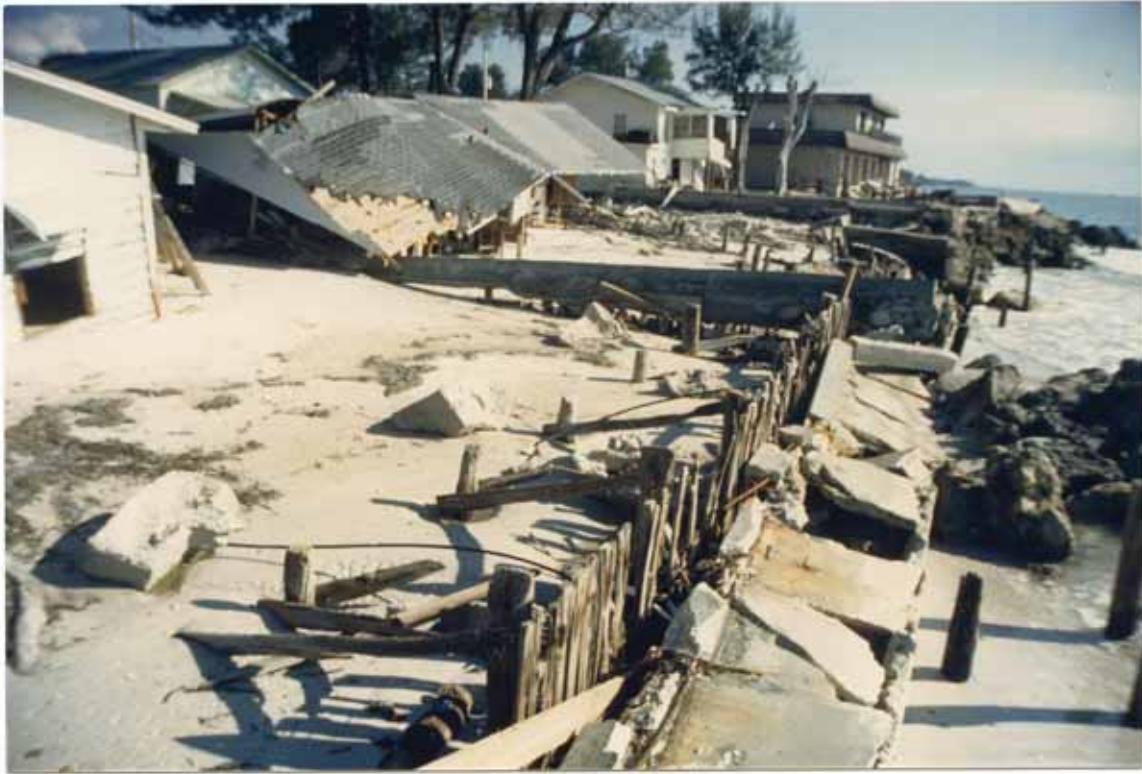
FIGURE 139. Bulkheads destroyed by wave loads
