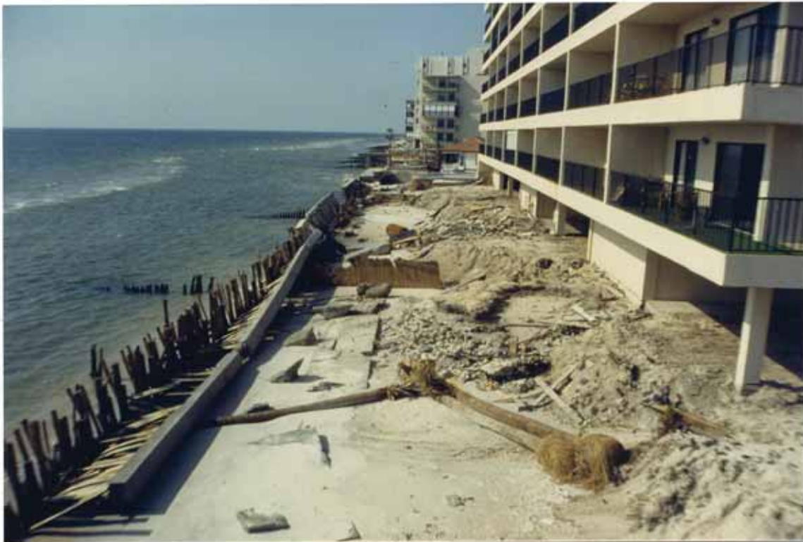
FIGURE 108. Indian Shores bulkheads destroyed, 820 feet
