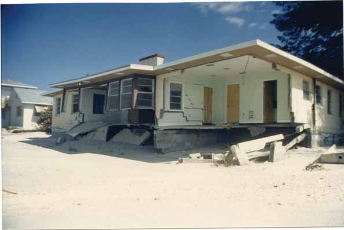
FIGURE 129. Juan's beach accretion at damaged dwelling
