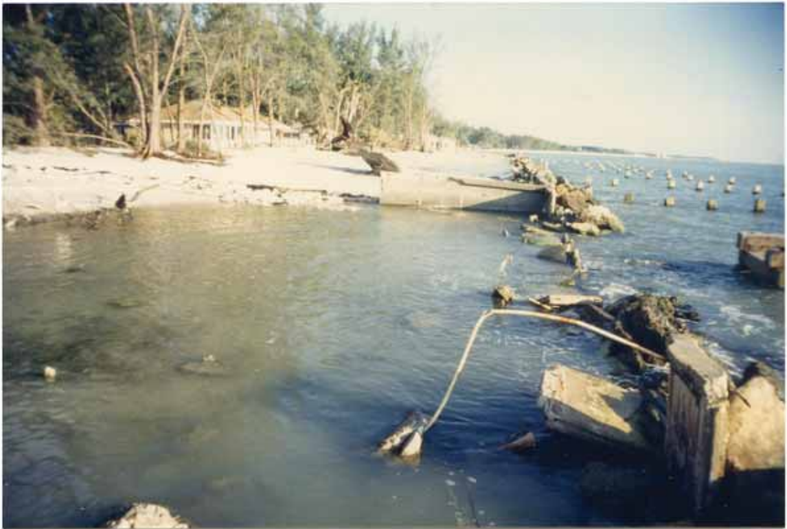
FIGURE 142. Juan destroyed 700 feet of bulkheads
