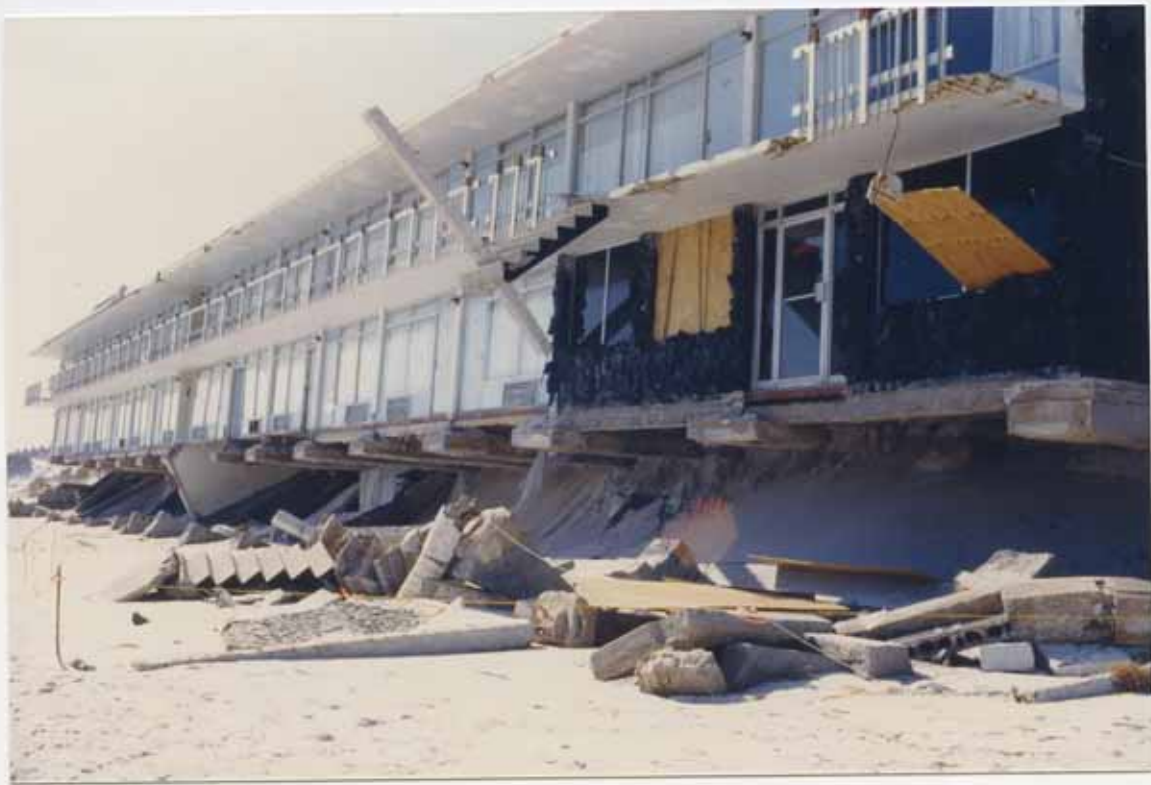
FIGURE 2. Dunes Motel damaged by Elena's erosion, Pensacola Beach (D. Dodder)
