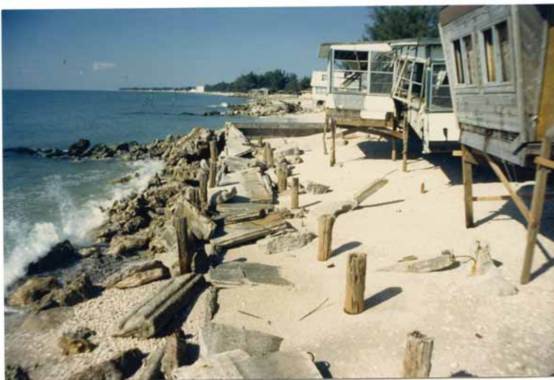
FIGURE 134. Bulkhead with toe-scour protection destroyed
