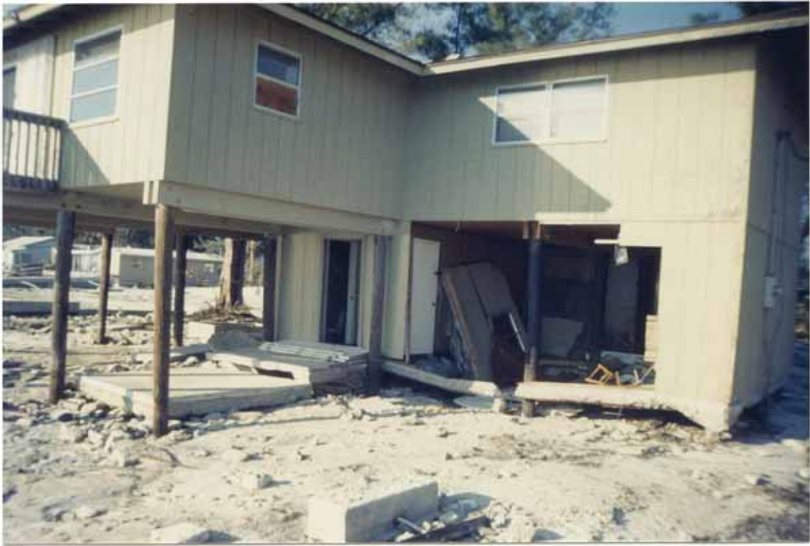
FIGURE 141. Subfloor damage to Longboat Key dwelling
