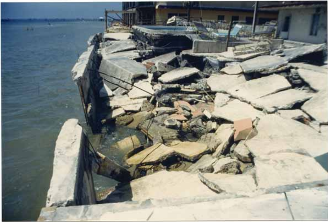
FIGURE 119. Flagship property damage after Elena
