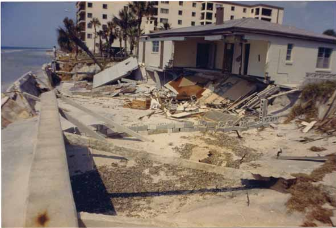
FIGURE 72. Dwelling damaged by Elena
