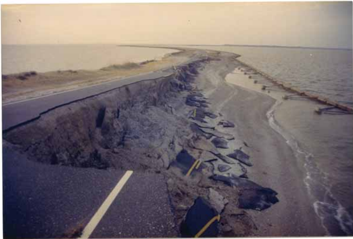
FIGURE 15. St. George Island causeway damaged by Elena's waves
