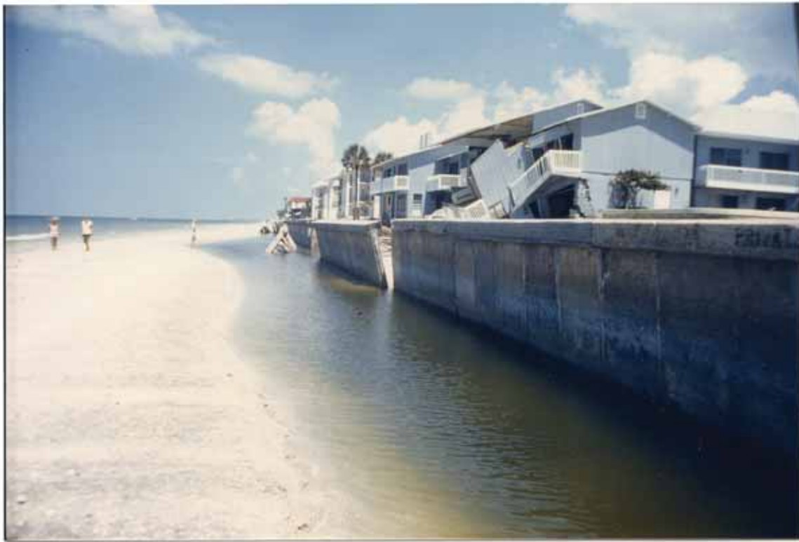
FIGURE 60. Bulkhead damage, La Casa de los Caracoles, Belleair Beach
