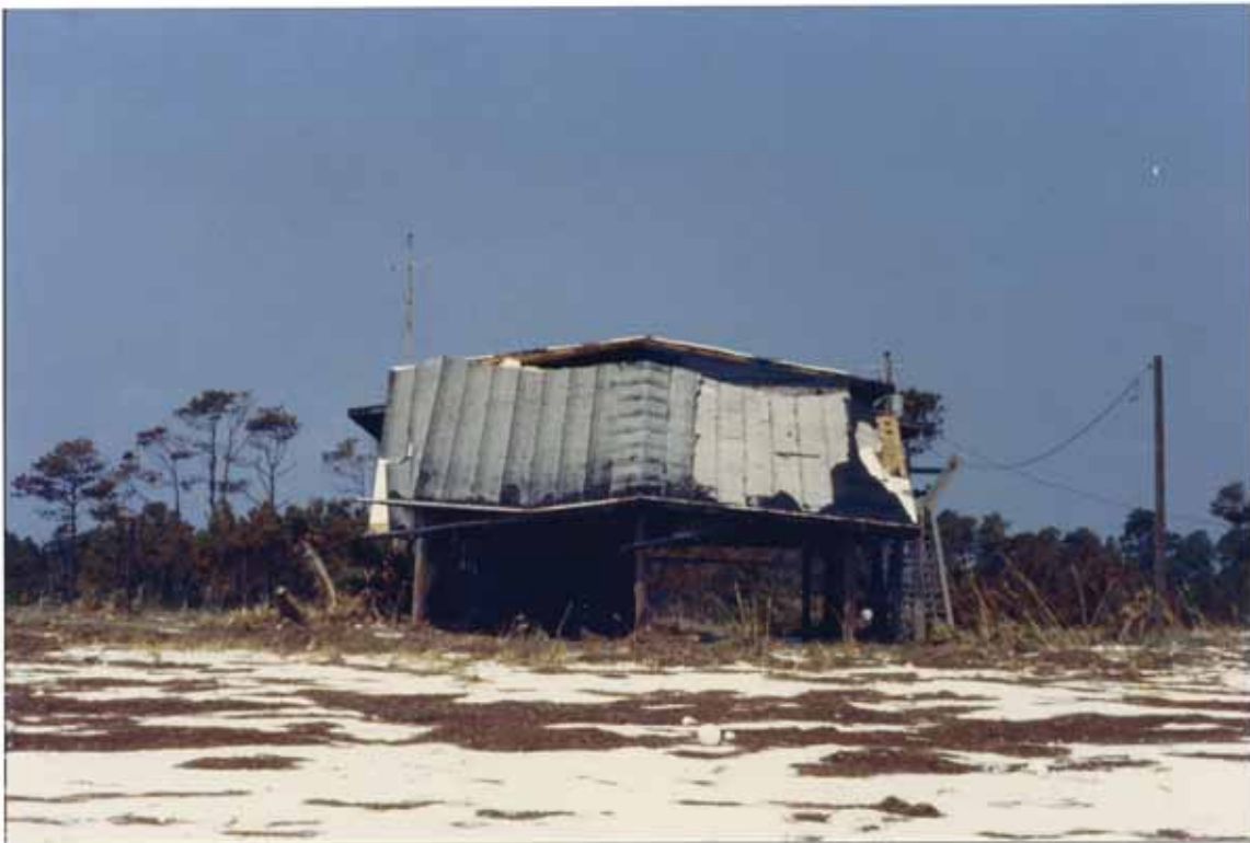
FIGURE 11. Dwelling damaged by Elena's wind, Dog Island (G. L. Hill)
