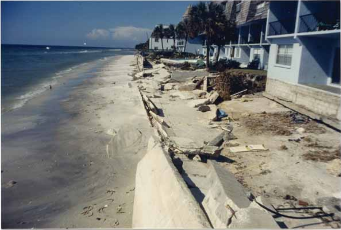
FIGURE 97. Happy Fiddler Condominium bulkhead after Elena
