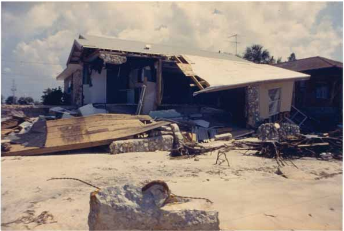
FIGURE 85. Dwelling damaged by Elena
