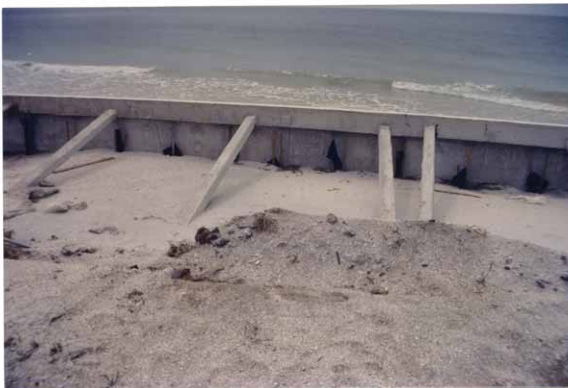
FIGURE 59. Inadequate fill containment with strips of filter fabric
