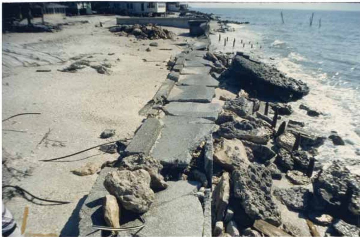
FIGURE 132. Bulkhead destroyed by wave impact loads
