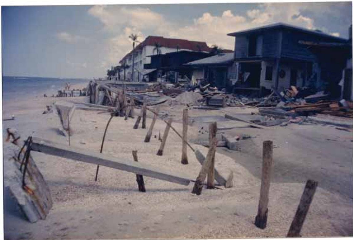
FIGURE 55. Concrete bulkhead destroyed by Elena, Belleair Beach
