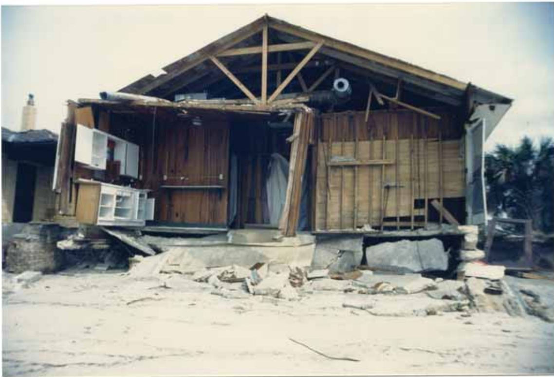
FIGURE 87. Same dwelling damaged by Juan
