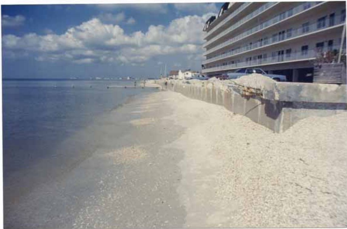
FIGURE 123. Juan damaged Sunset Chateau Condominium's bulkhead, Treasure Island
