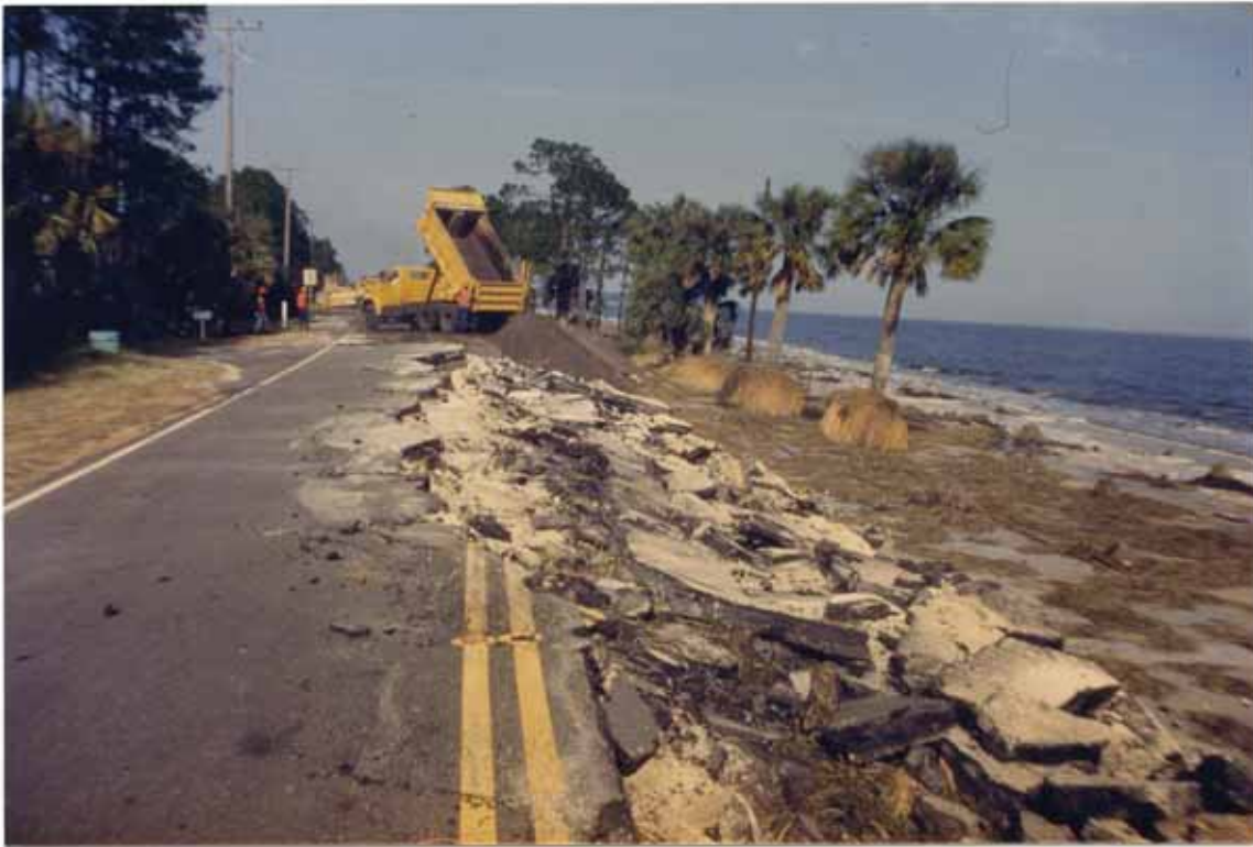
FIGURE 16. U.S. Highway 98 damaged by Elena, Carrabelle Beach
