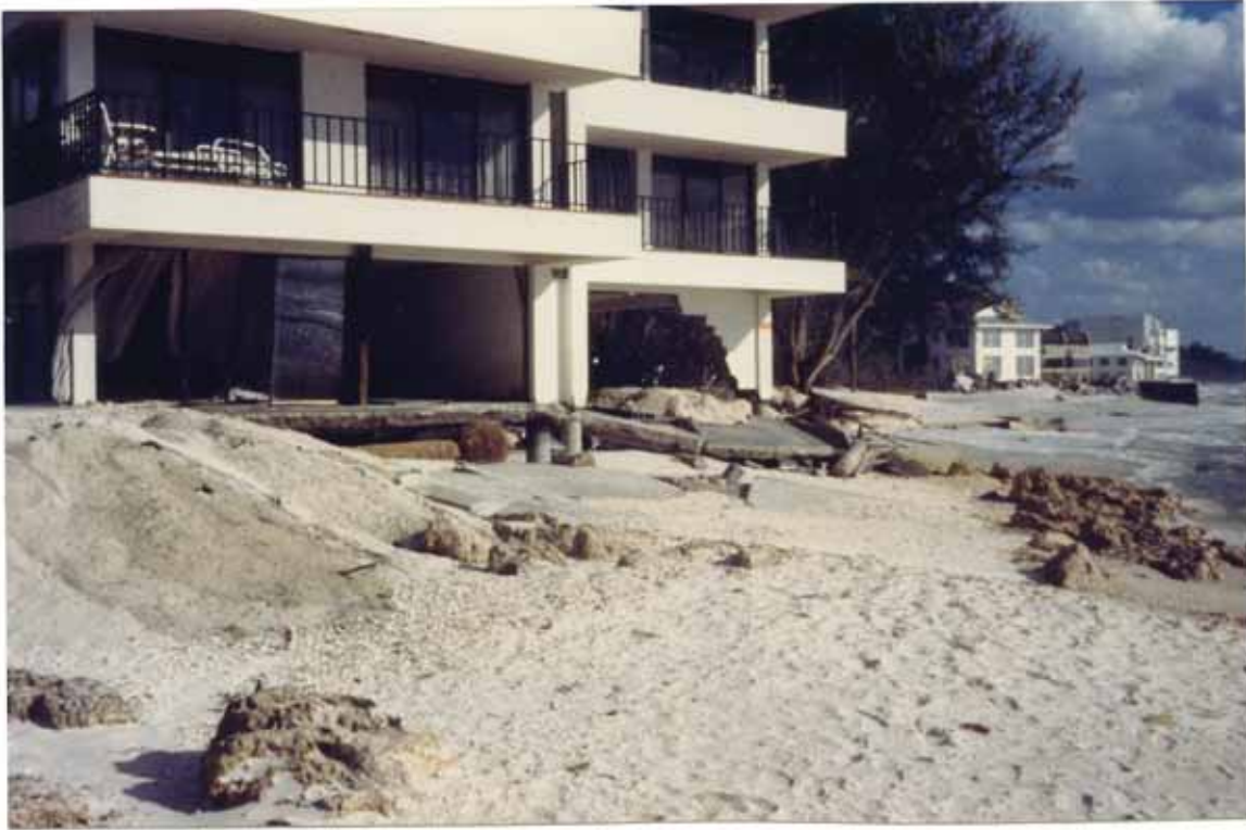
FIGURE 125. Waters Edge Condominium damaged by Elena (S. West)
