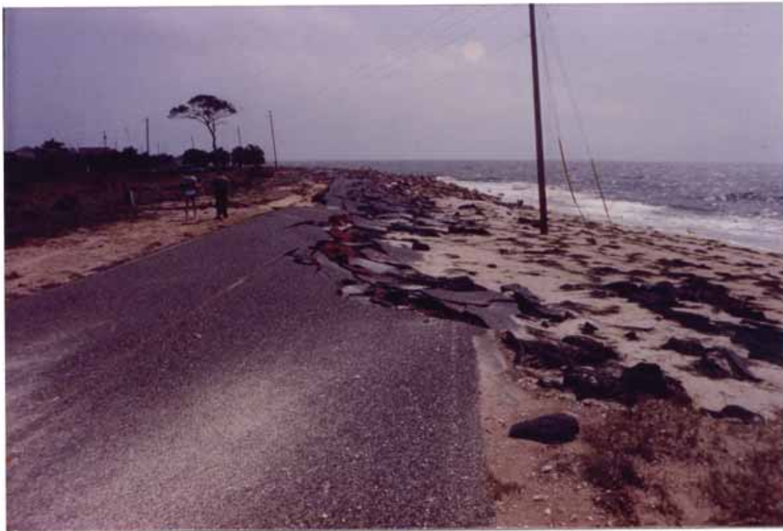
FIGURE 31. Elena's second pass destroyed County Road C370 on September 1
