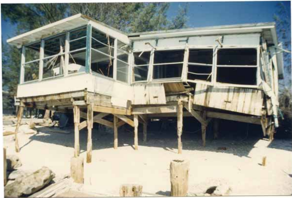
FIGURE 135. Holmes Beach dwelling destroyed by Elena
