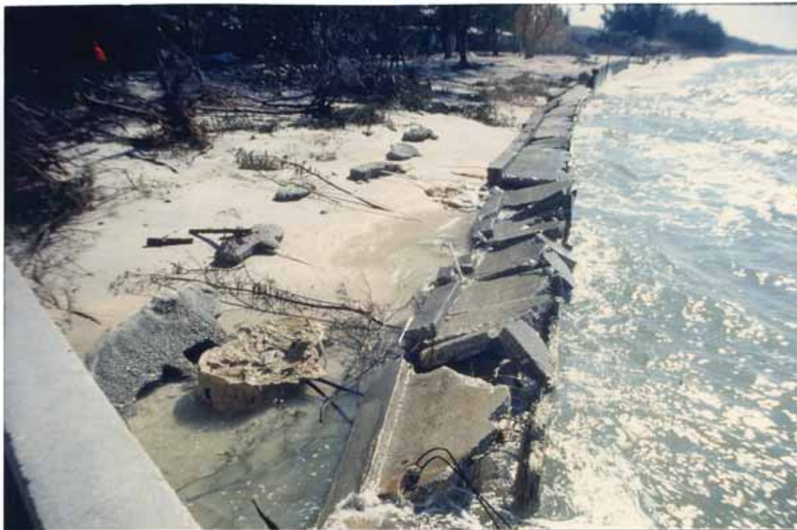
FIGURE 127. Elena and Juan destroyed 920 feet of bulkhead
