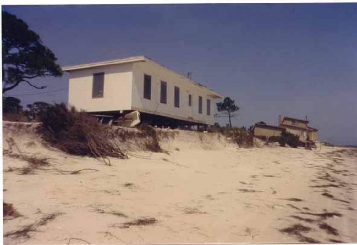
FIGURE 41. Lighthouse Point dwelling threatened by Elena's erosion
