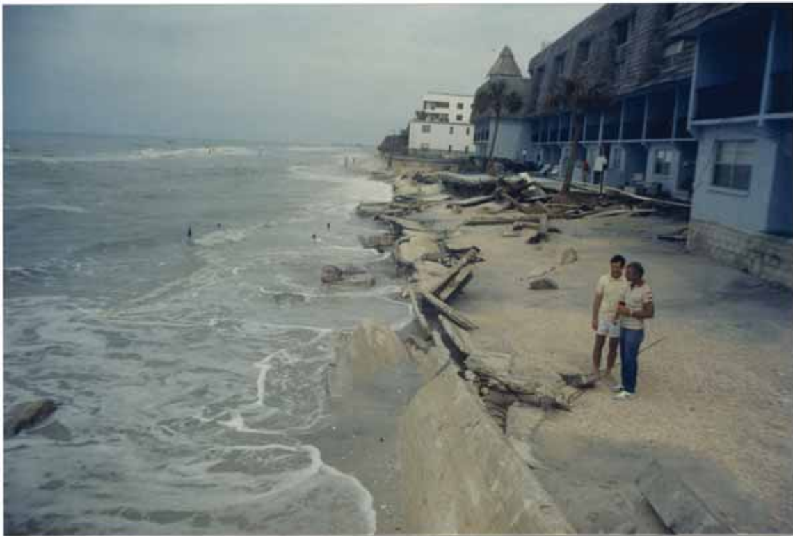
FIGURE 98. Happy Fiddler Condominium bulkhead after Juan
