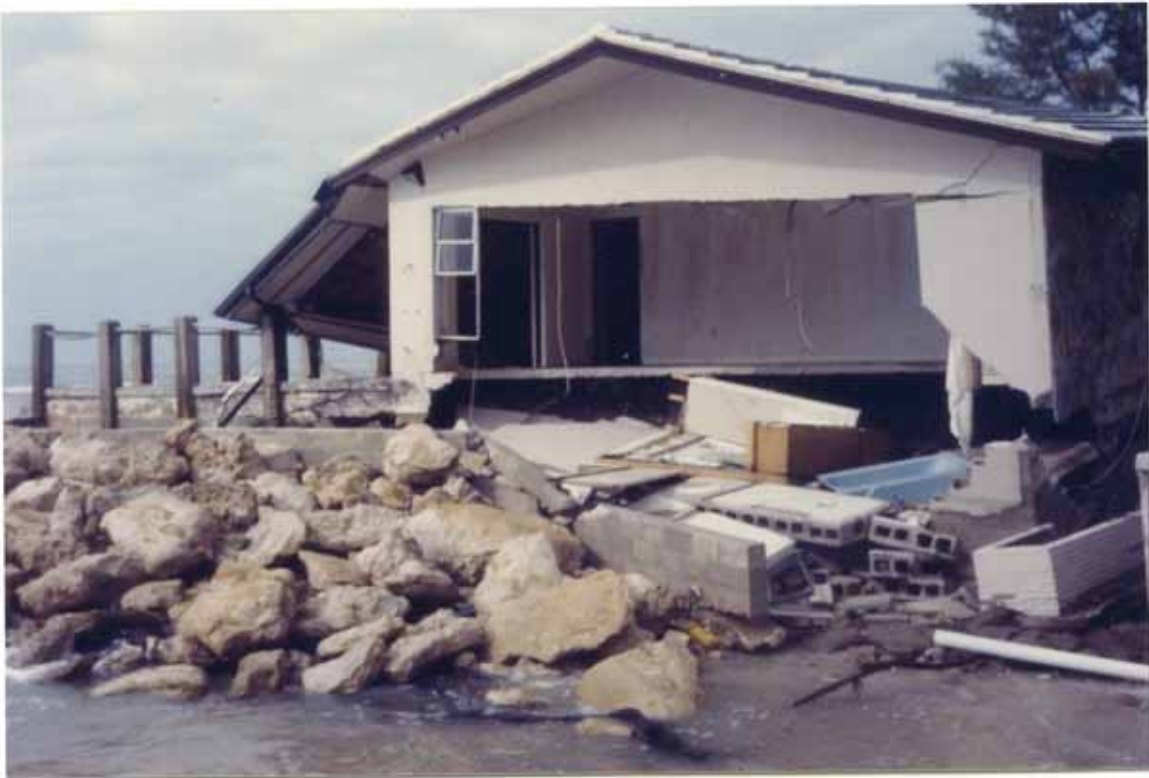
FIGURE 144. Same dwelling destroyed by wave flanking (M. Joity)
