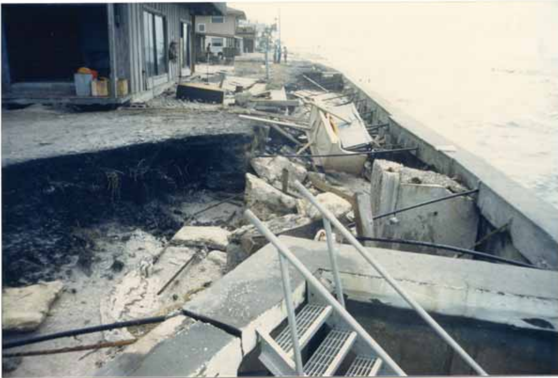
FIGURE 95. Juan eroded street-end fill, 7th Avenue
