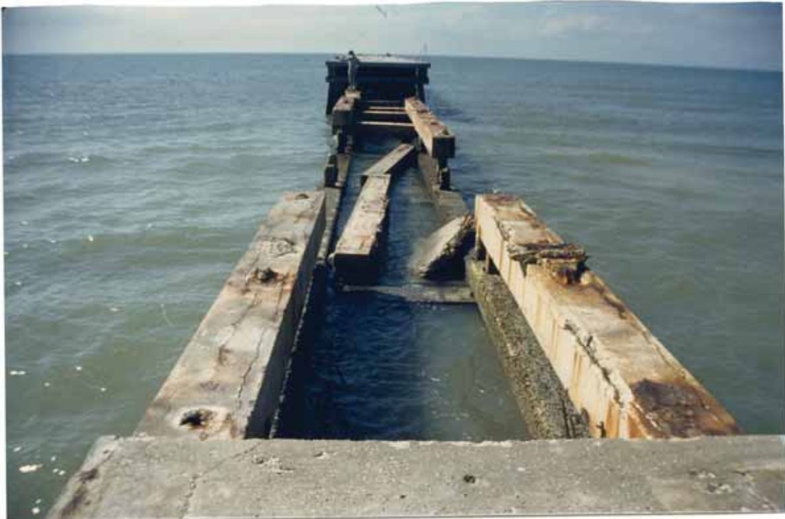
FIGURE 130. Juan damaged pier-groin at County park
