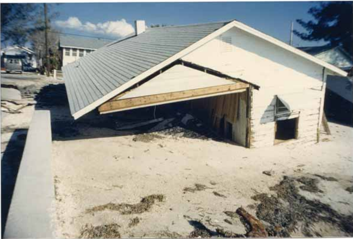
FIGURE 138. Same dwelling destroyed by Juan
