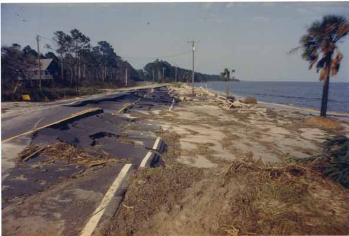
FIGURE 17. U.S. Highway 98 damaged by Elena
