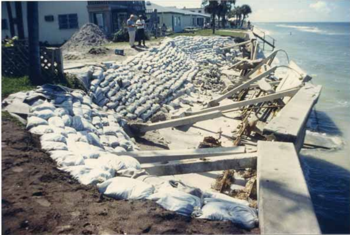
FIGURE 75. Post-Elena emergency protection, 23rd Avenue
