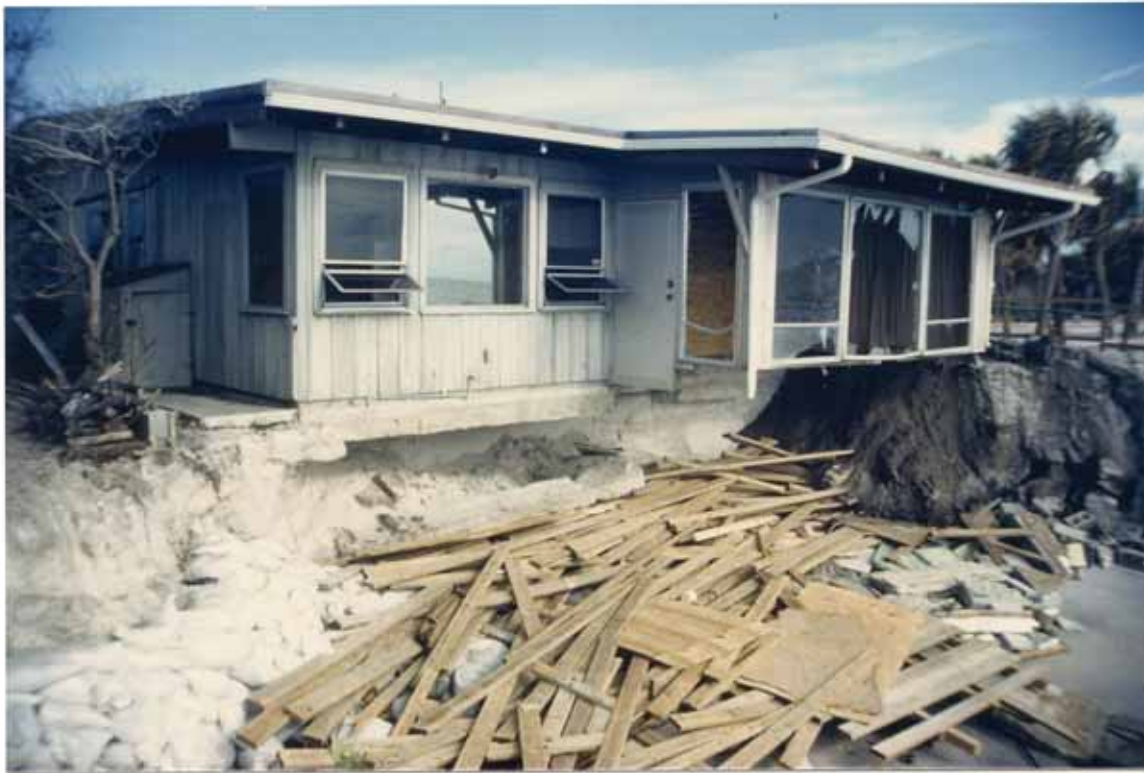
FIGURE 117. Redington Shores dwelling damaged by Juan
