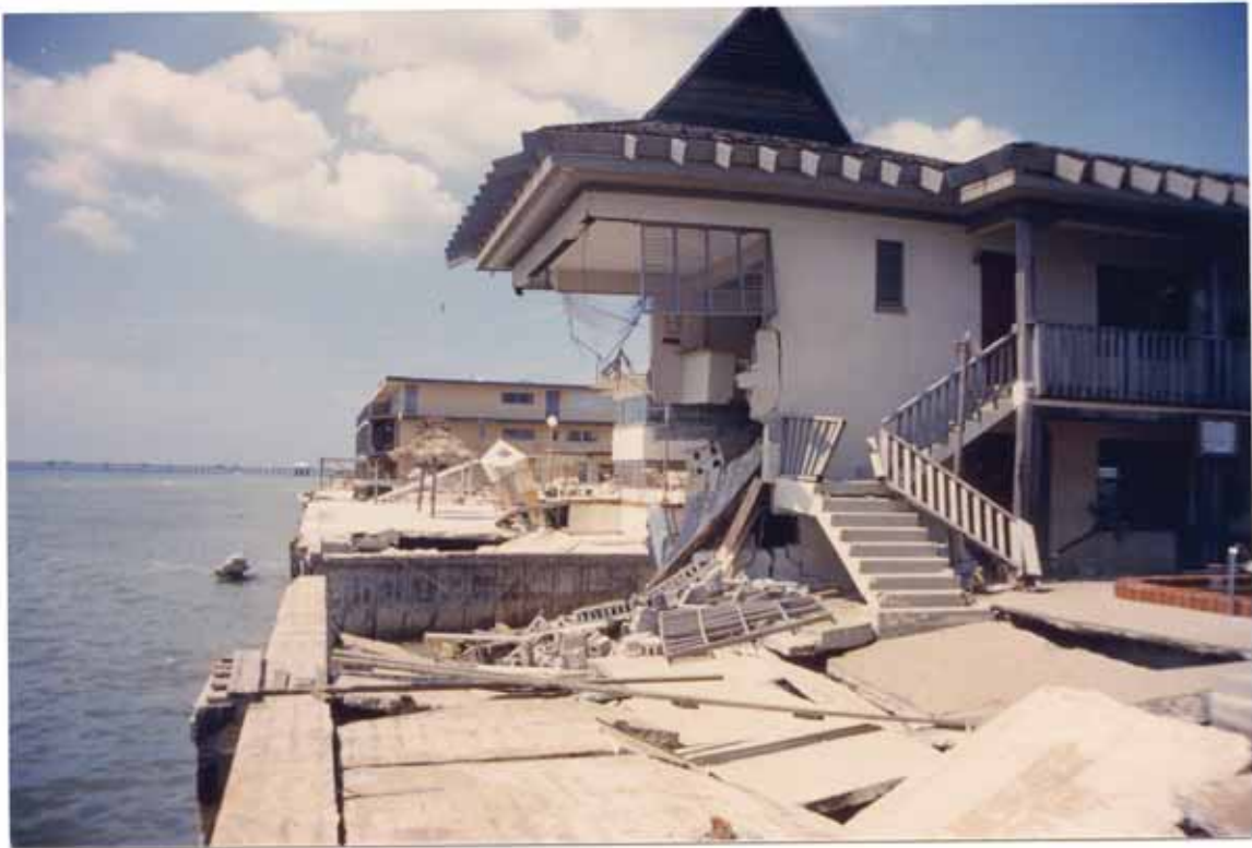
FIGURE 121. The Islander after Elena's damage
