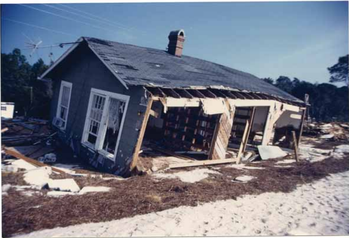
FIGURE 19. Carrabelle Beach dwelling destroyed by Elena
