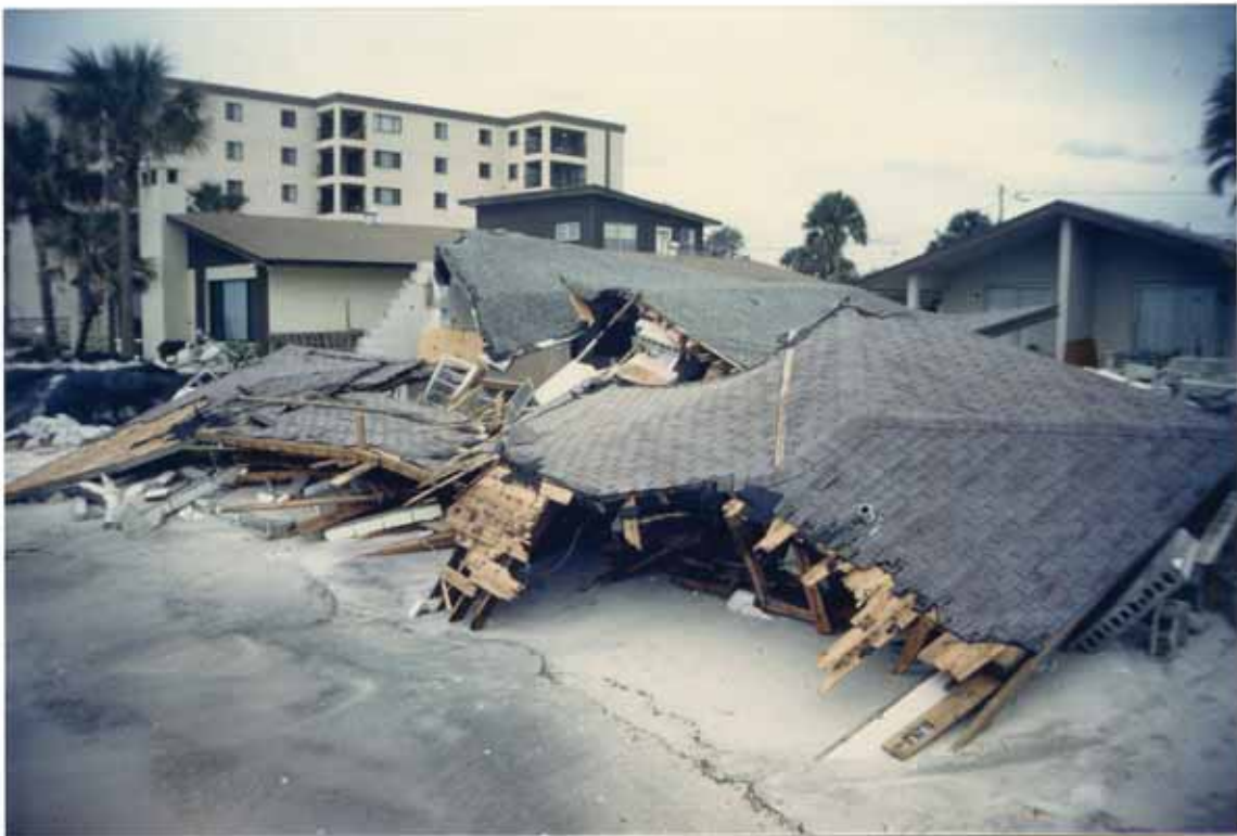
FIGURE 71. Dwelling destroyed by Juan
