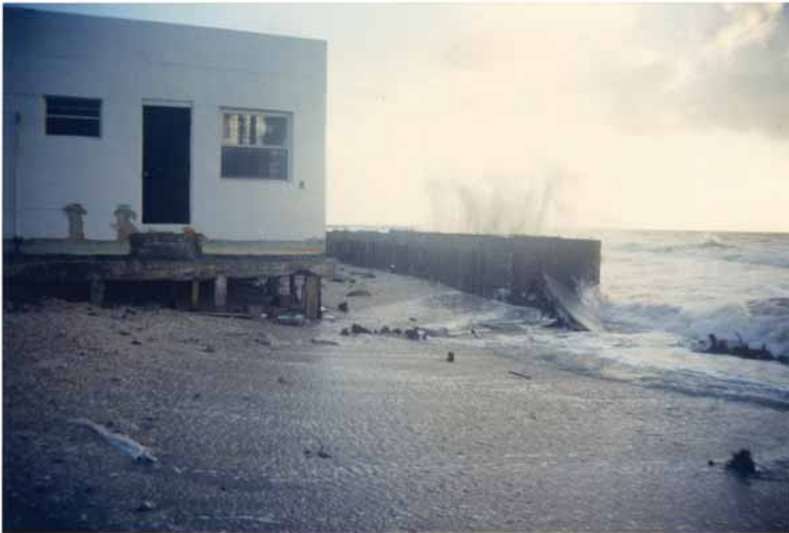
FIGURE 110. New bulkhead damaged without toe-scour protection
