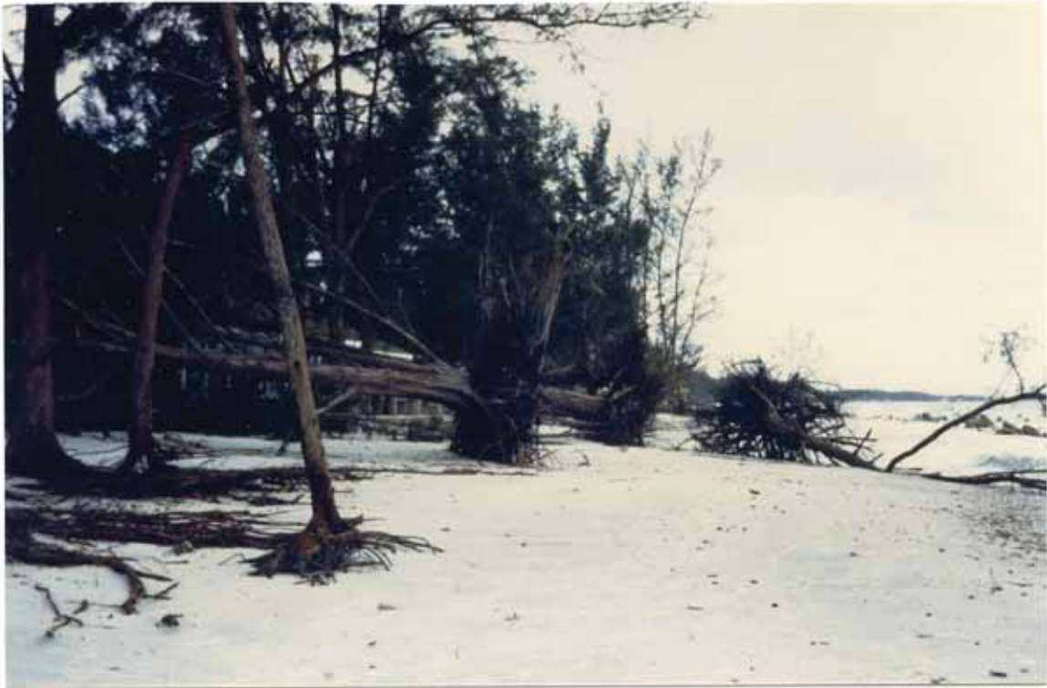
FIGURE 145. Severe erosion on Longboat Key (S. West)
