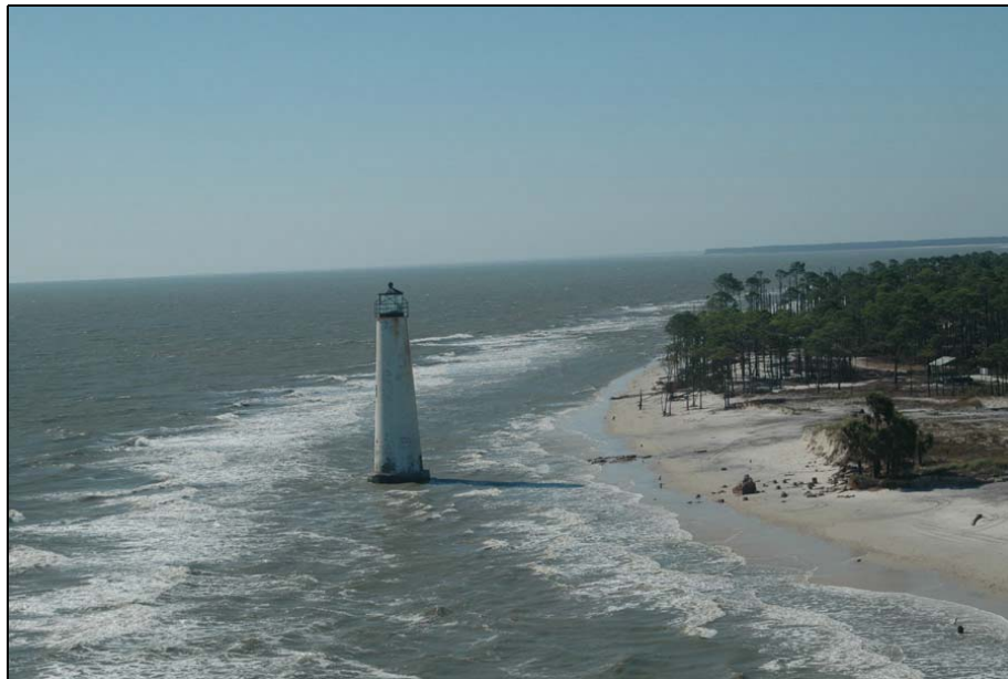
Photo FR-1. View of Cape St. George lighthouse after Ivan (note: the lighthouse was substantially seaward of the shoreline into Gulf waters prior to Ivan).
