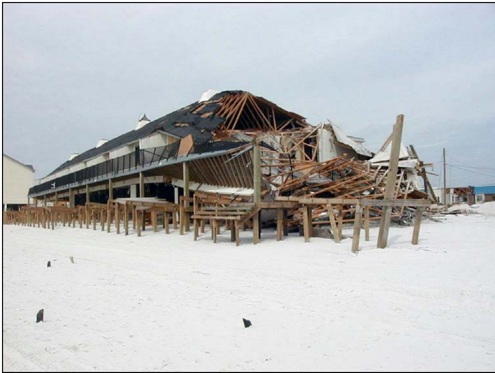
Photo ES-11. Destroyed multi-family dwelling at R116 (+300') in Pensacola Beach.
