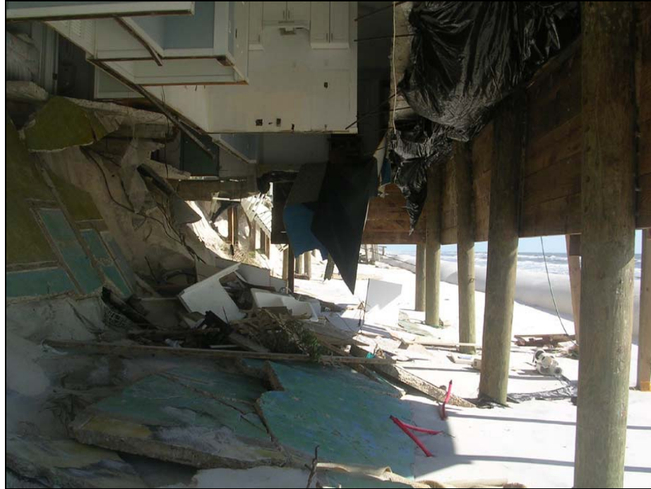
Photo GU-7. Sand loss and collapse of floor beneath habitable structure on St. Joseph Peninsula at R83 (+500').
