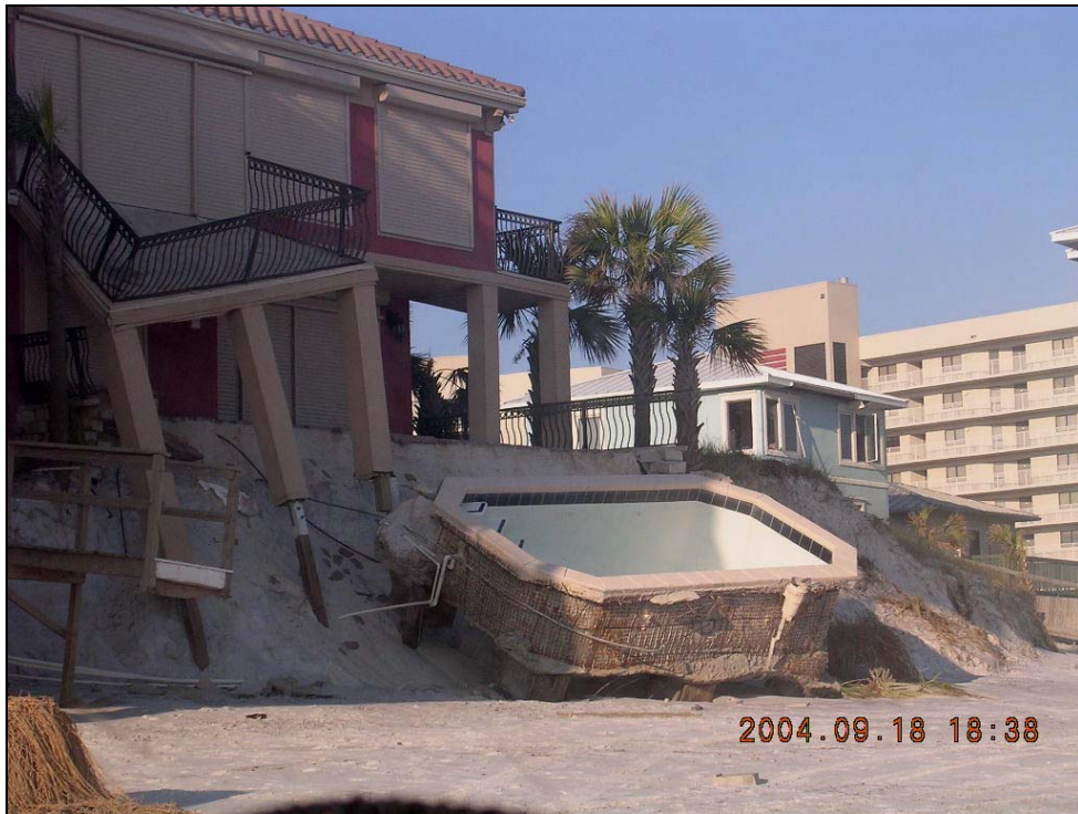
Photo WL-3. Erosion and destroyed swimming pool near R9.
