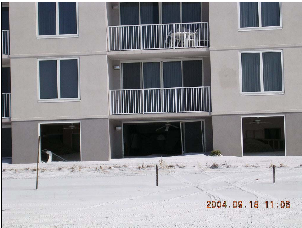
Photo OK-2. Overwash sand deposition and flooding damage in bottom floor areas near R1.
