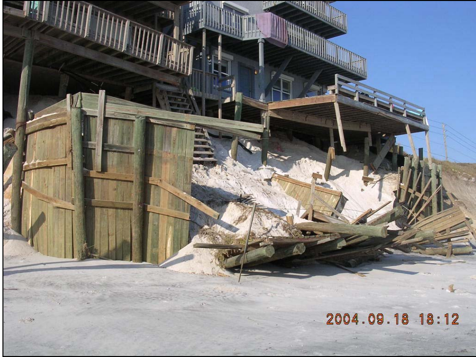
Photo WL-2. Destroyed retaining wall near R9.
