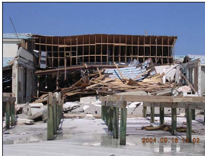
Photo OK-4. Destroyed beach club building; Eglin Air Force Base; east Santa Rosa Island
