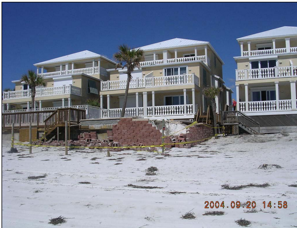
Photo BA-4. Damage to block retaining wall at R76 (+200) in Panama City Beach.
