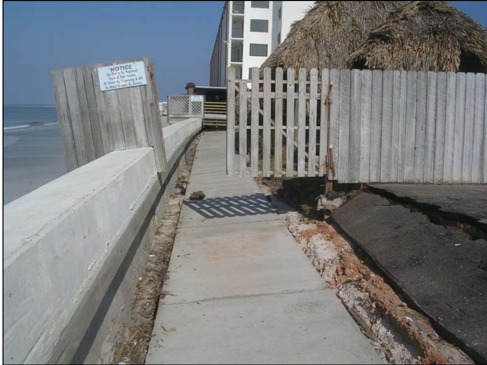
Photo BA-7. Damage to the El Governor seawall in Mexico Beach at R135 (-300').
