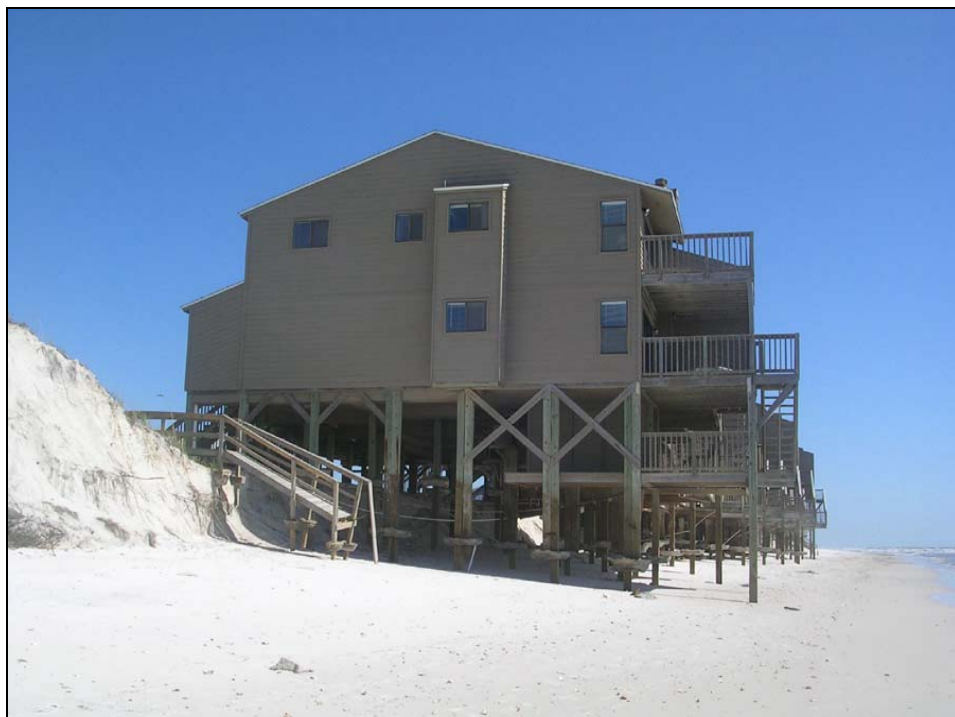
Photo GU-6. Major dune erosion at habitable structures on the beach on St. Joseph Peninsula at R90 (+300').
