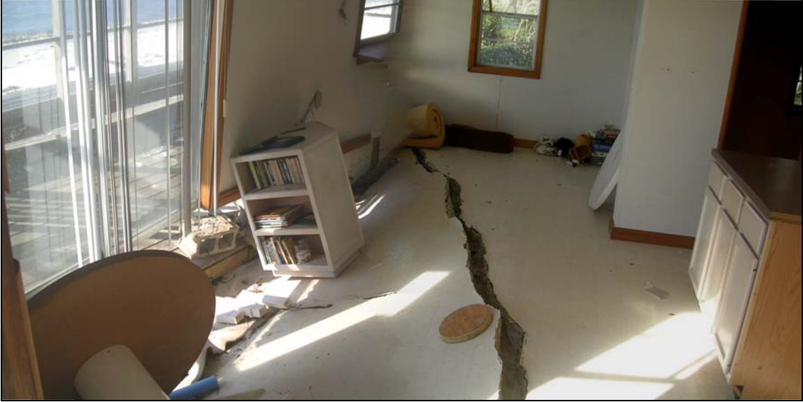
Photo FR-4. Major damage to single-family structure at Lighthouse Point at R221 (+50').
