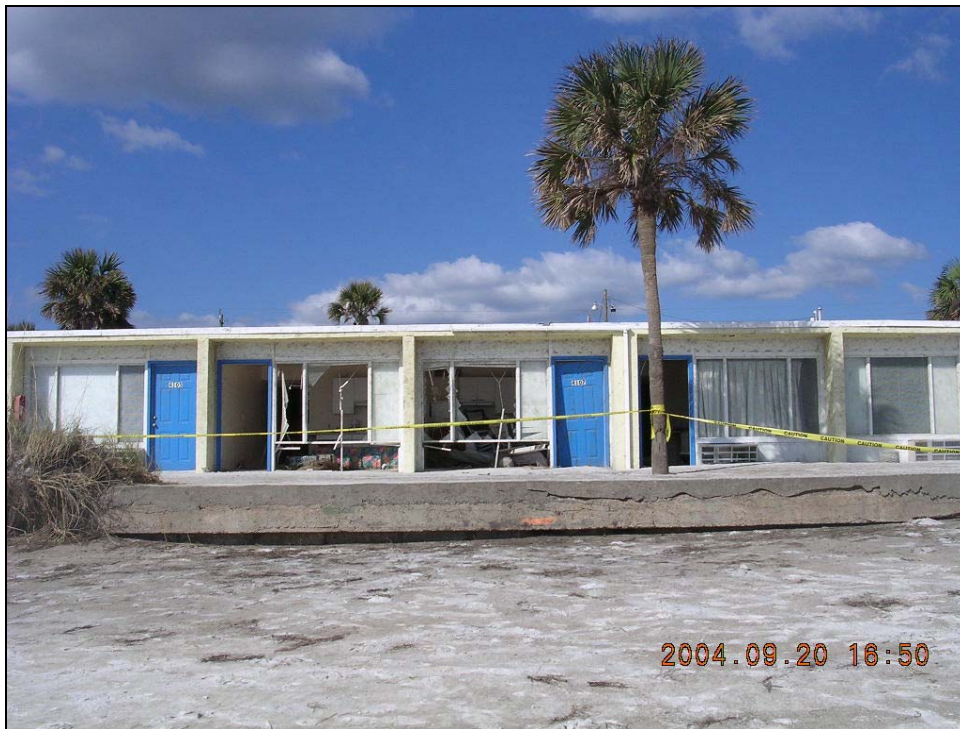
Photo BA-2. Major damage to motel structure at R22 (-400') in Bay County.
