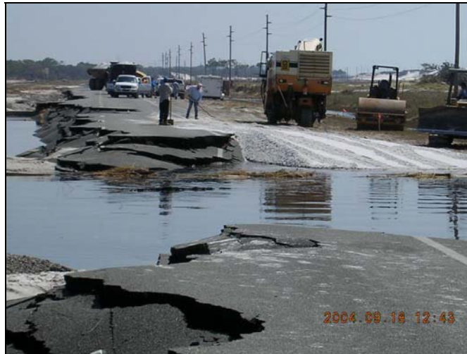
Photo OK-3. Damage to Highway 98 between Destin and Ft. Walton Beach.
