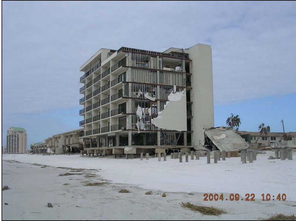
Photo SR-5. Multi-family dwelling with major damage near R208 in Navarre Beach.
