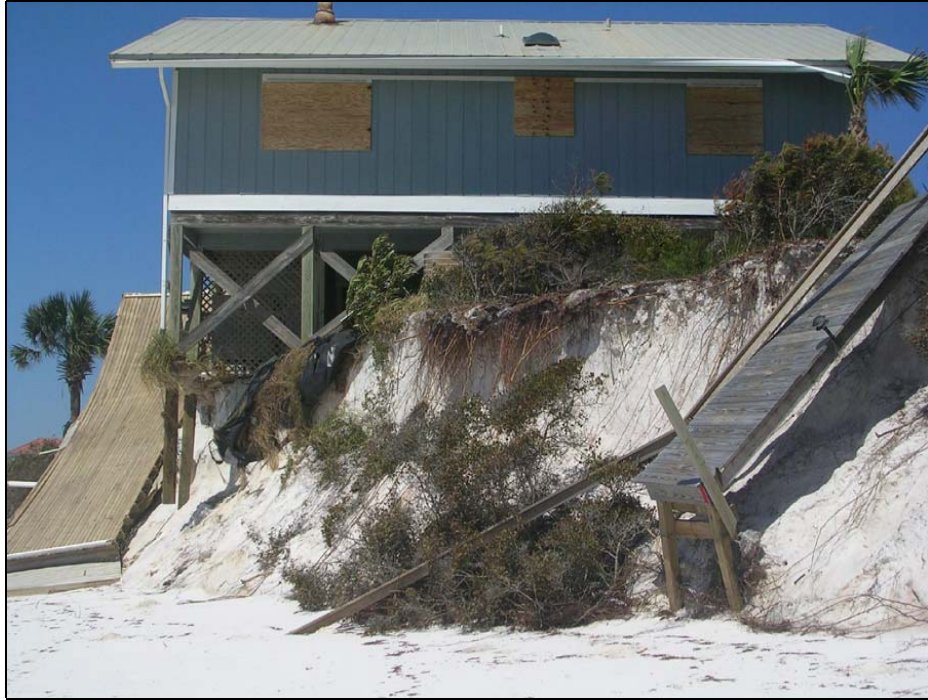
Photo GU-5. Eroded dune bluff; structural damage at R99; St. Joseph Peninsula
