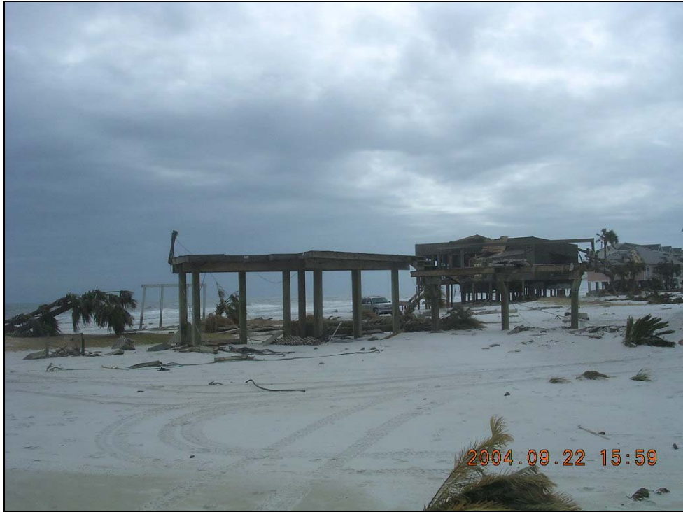
Photo ES-19. Remains of destroyed single-family dwelling; R137 (+100'), Pensacola Beach.
