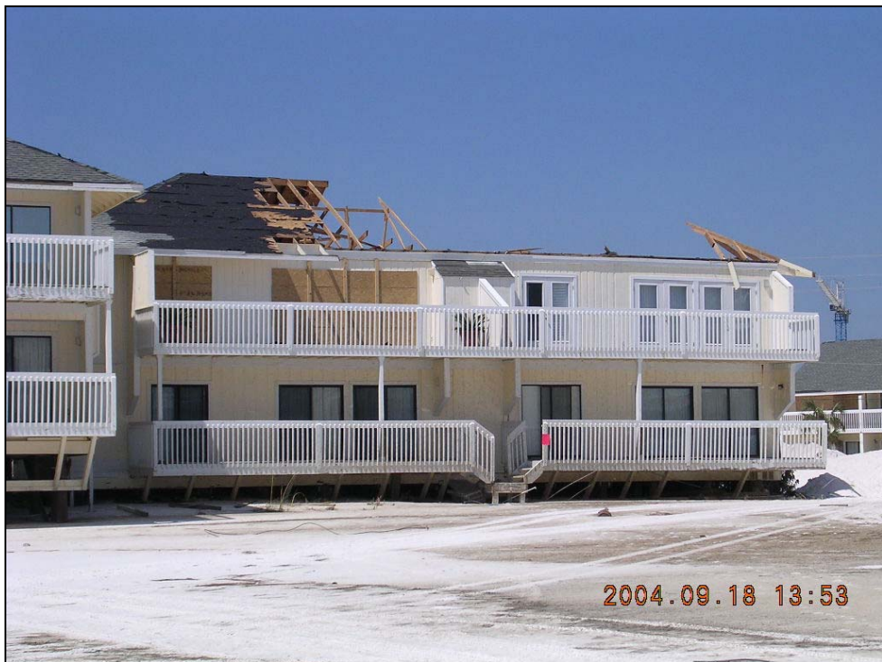
Photo OK-9. Major habitable structure damage in Destin between R24-25.
