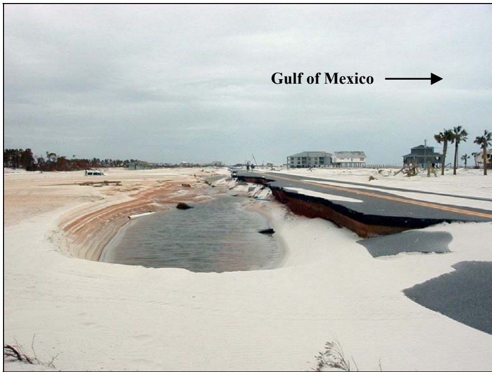
Photo ES-2. Damage to Perdido Key Dr. (C.R. 292) between R11 and R13 on Perdido Key.
