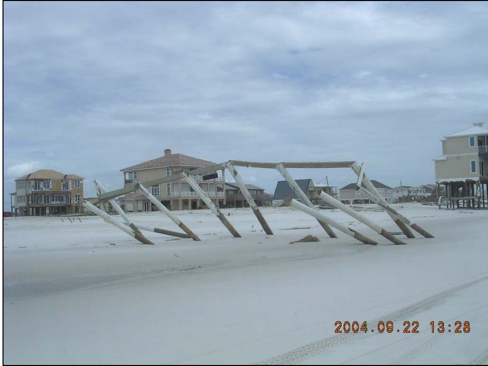
Photo SR-1. Remains of destroyed single-family dwelling at R194 (-100') in Navarre Beach.
