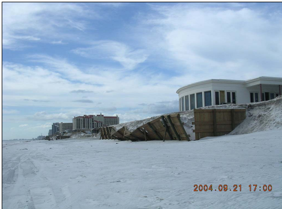
Photo WL-5. Destroyed retaining wall at location R23 (+500').
