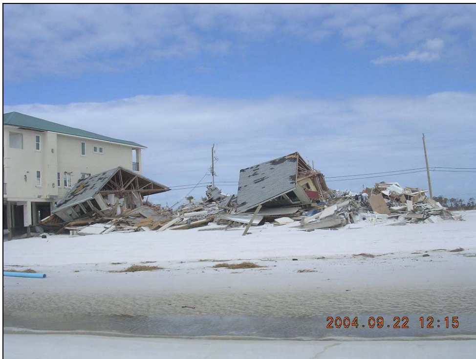
Photo SR-2. Destroyed single-family dwellings near R200 (+700') in Navarre Beach adjacent to better designed dwelling that survived major damage from Ivan.
