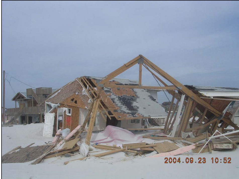
Photo ES-12. Destroyed single-family dwelling at R125 (+350') in Pensacola Beach.
