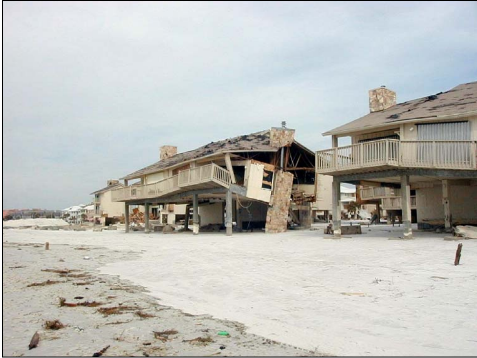
Photo ES-10. Destroyed single-family dwelling at R111 (-200') in Pensacola Beach.
