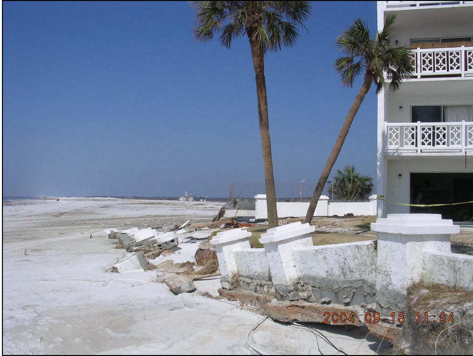
Photo OK-1. Damage to decorative wall and lower floor on Okaloosa Island near R1.
