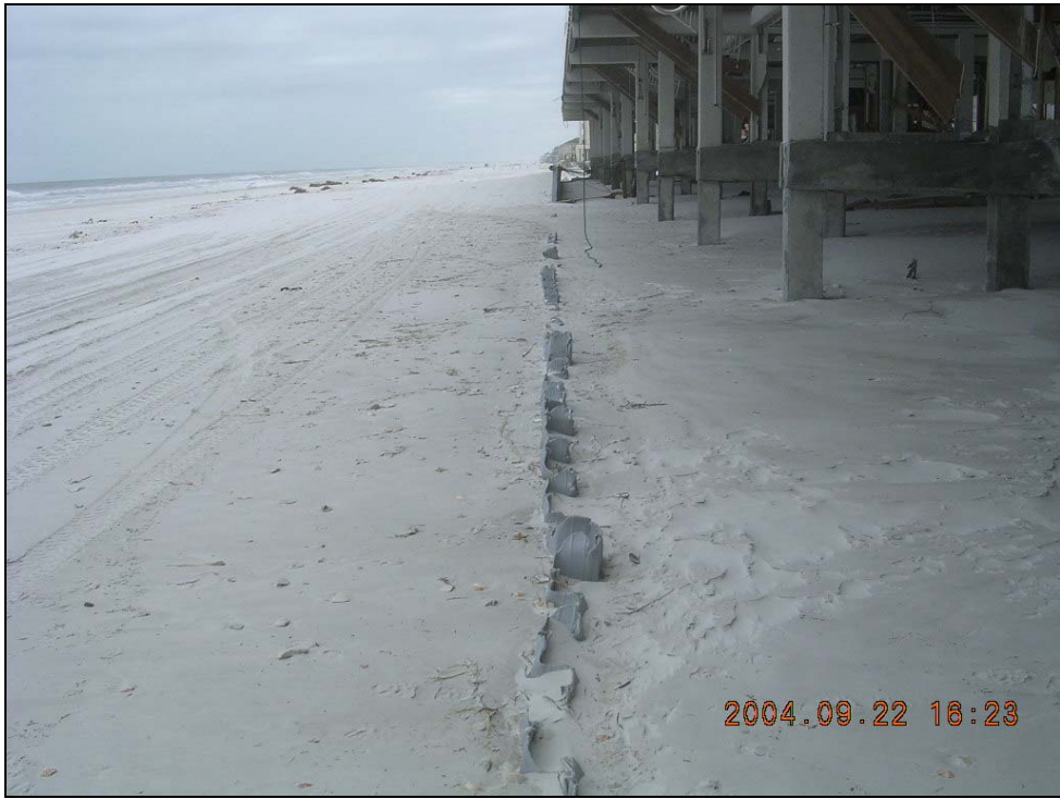
Photo ES-15. Destroyed sheet-pile wall sheared off at eroded grade elevation; R136 (+250').
