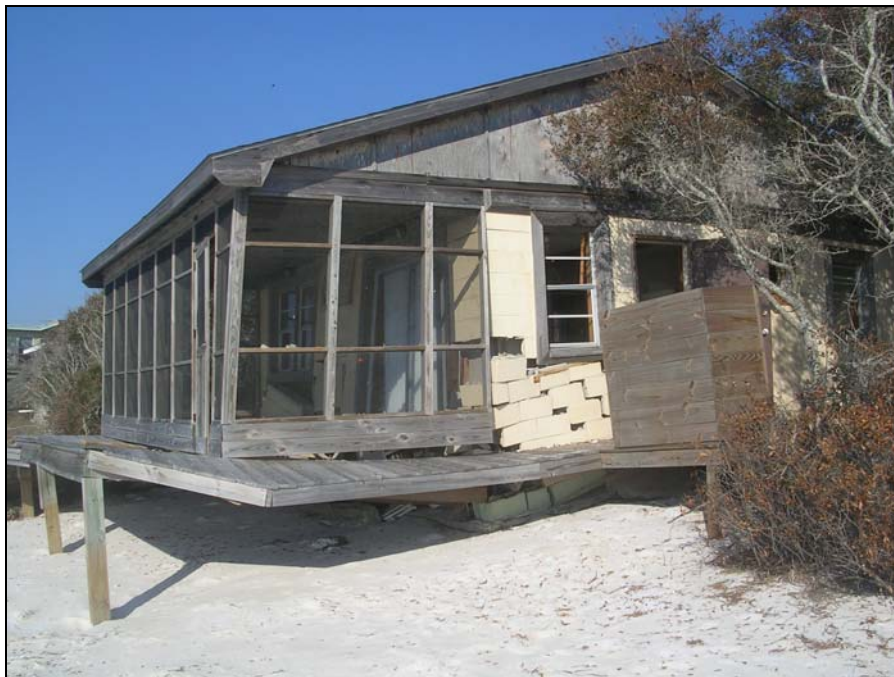
Photo FR-3. Destroyed single-family structure at Lighthouse Point at R221 (+50').
