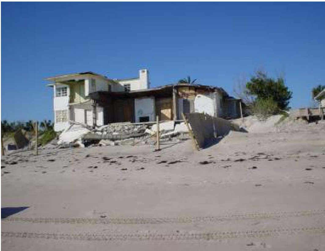
Photo 83. Foundation damage to single-family dwelling, Vero Beach (R79.5).
