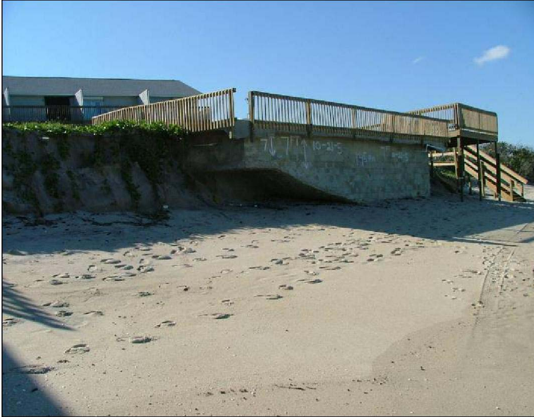
Photo 84. Pool undermined by Hurricane Wilma, Brevard County (R158.5).
