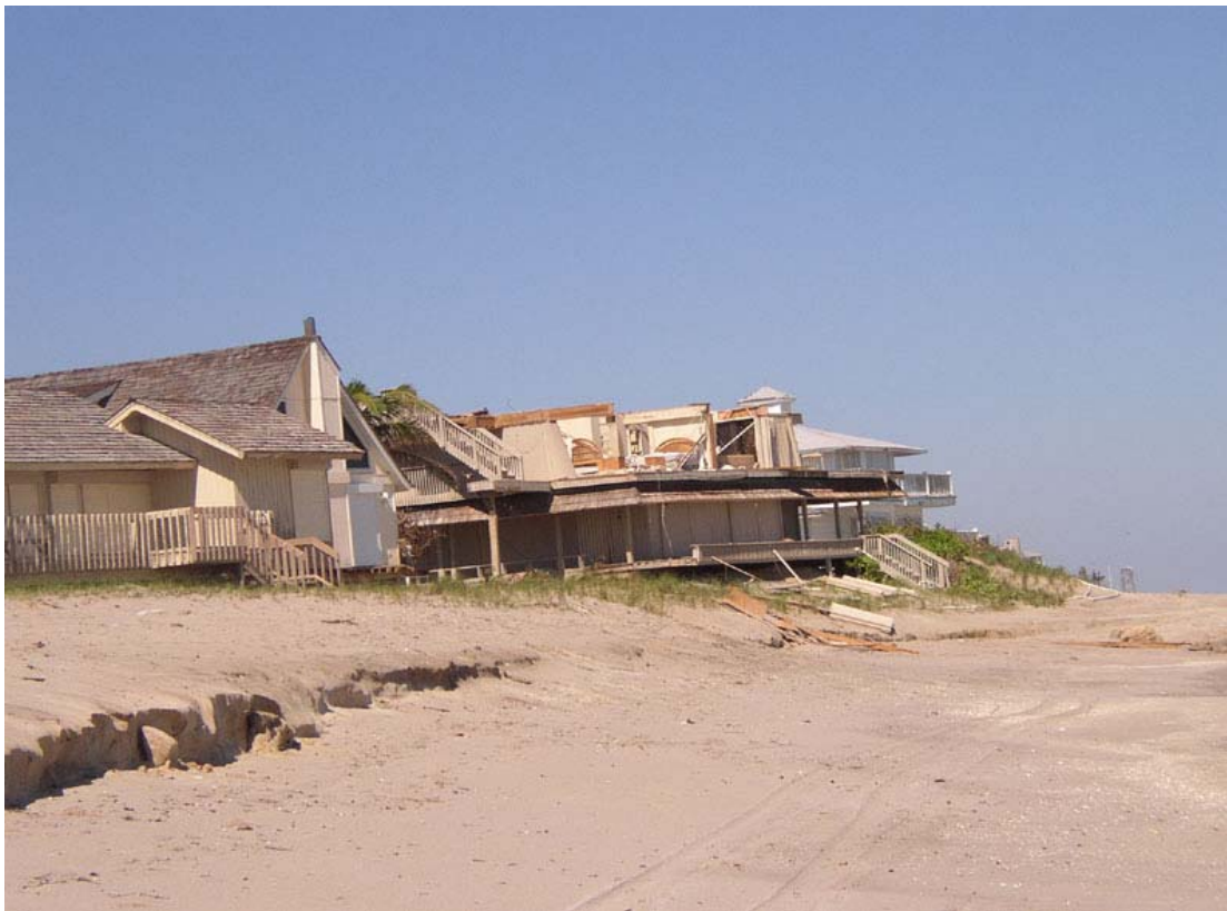
Photo 82. Destroyed single-family dwelling, Martin County (R33).
