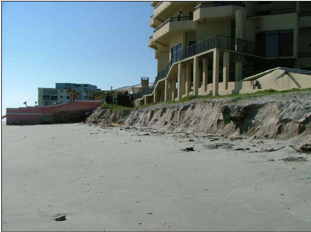
Photo 80. Severe dune erosion after Wilma at the Holiday Inn (R168).
