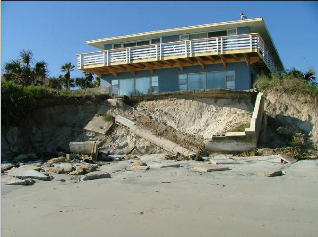
Photo 87. Patio and retaining wall destroyed, New Smyrna Beach (R167.3).
