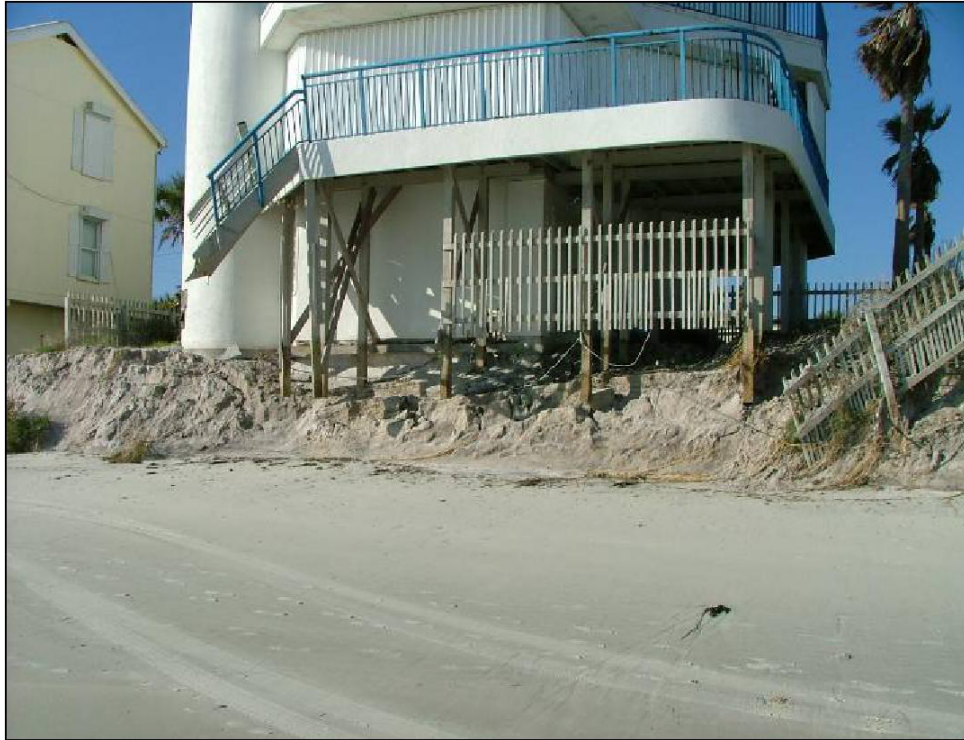
Photo 85. Undermined single-family dwelling, New Smyrna Beach (R160.8).
