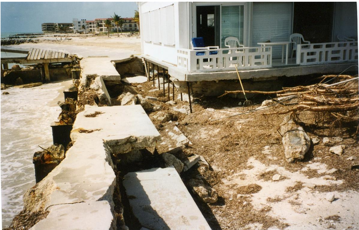
Damage at Key Colony Beach.
