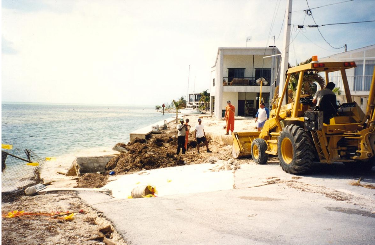
Damage at Geiger Key.
