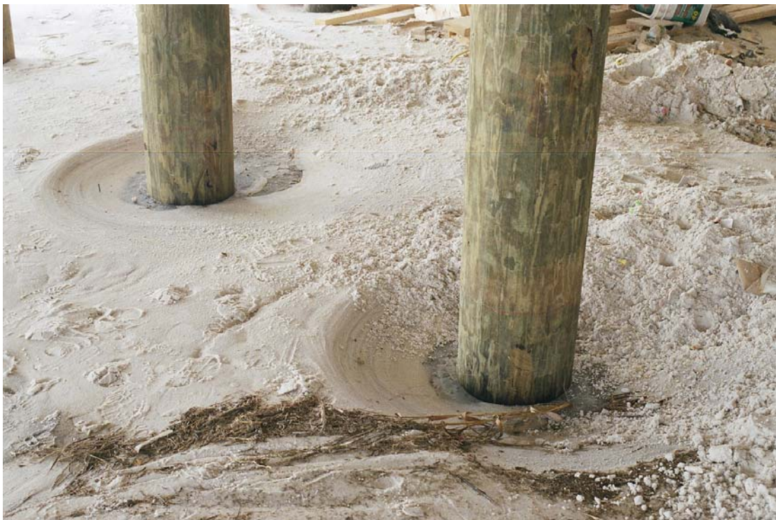
Photo 5. Typical localized pile scour [Photo from Chris Jones]
