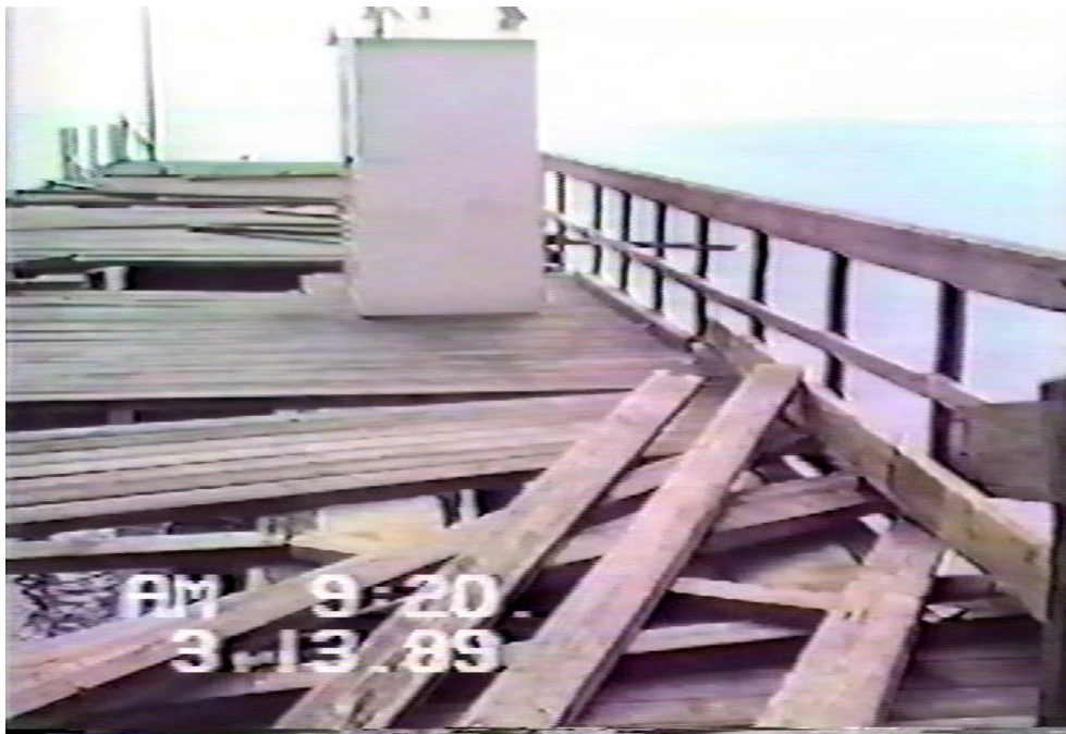
Photo 7. Pier decking damage, Lake Worth Pier (1972-2004) [BBCS Photo Files]
