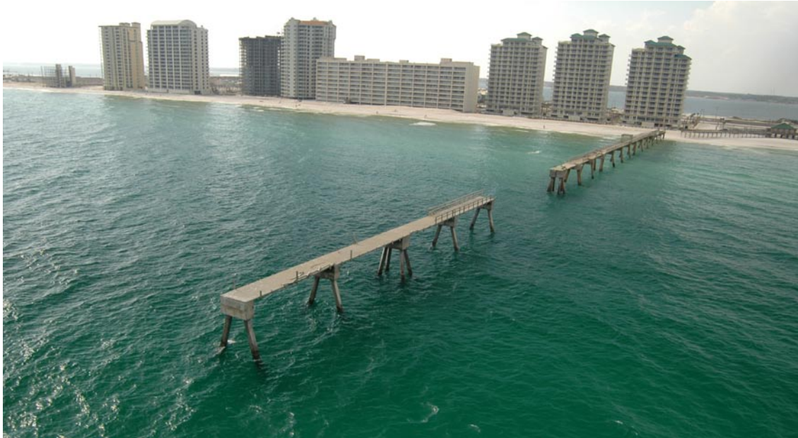
Photo 10. Hurricane Dennis destroyed three sections of the solid concrete Navarre Beach Fishing Pier at the seaward end, a mid-section, and at the shoreline [BBCS Photo Files]
