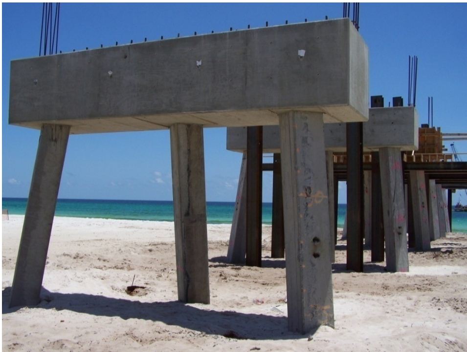
Photo 12. Concrete pile bent Russell-Fields Pier, Panama City Beach
