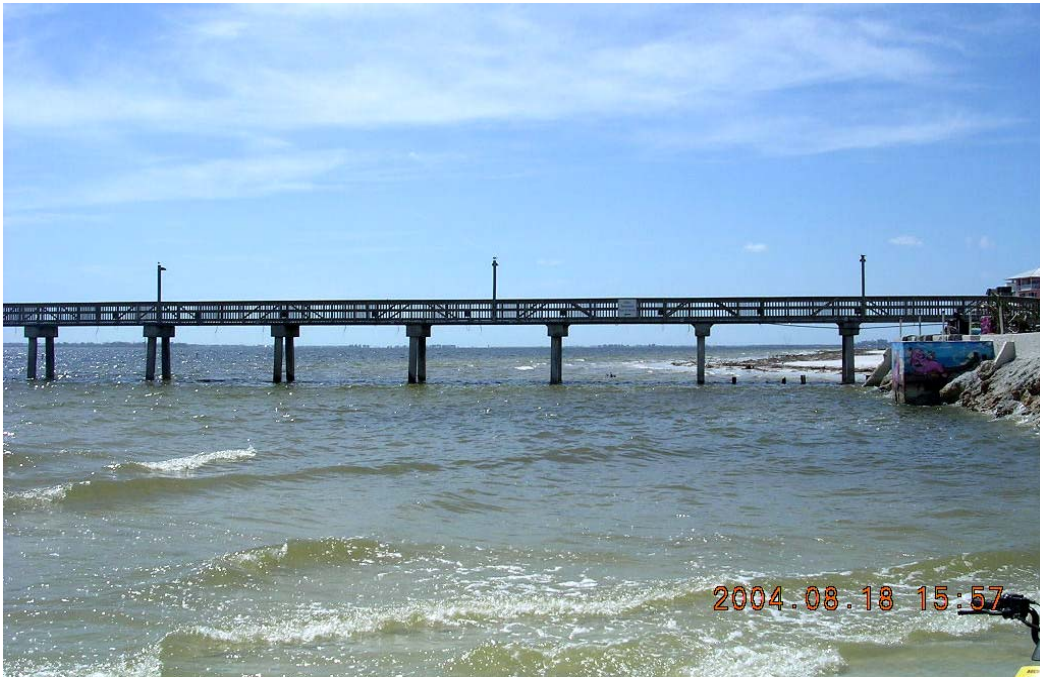
Photo 4. St. Augustine Beach Fishing Pier “fishable” again following the erosion of 2004 storms [BBCS Photo Files]
