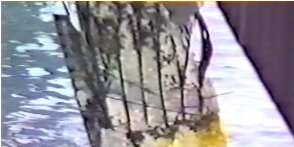
Photo 19. Concrete pile damage exposing deteriorated reinforcing steel [BBCS Photo Files]
