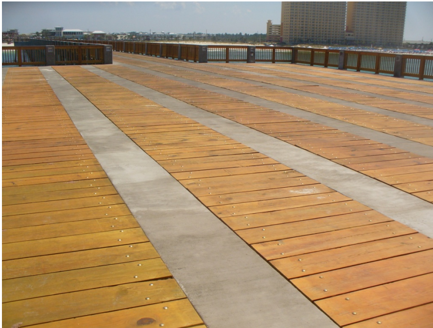
Photo 25. Breakaway wood deck at outer T-section, Russell-Fields Pier
