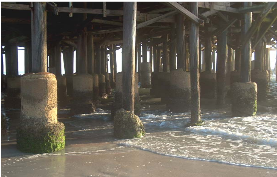
Photo 24. Concrete collars with bio-fouling, Daytona Beach Pier [Photo by John McDowell, BBCS]
