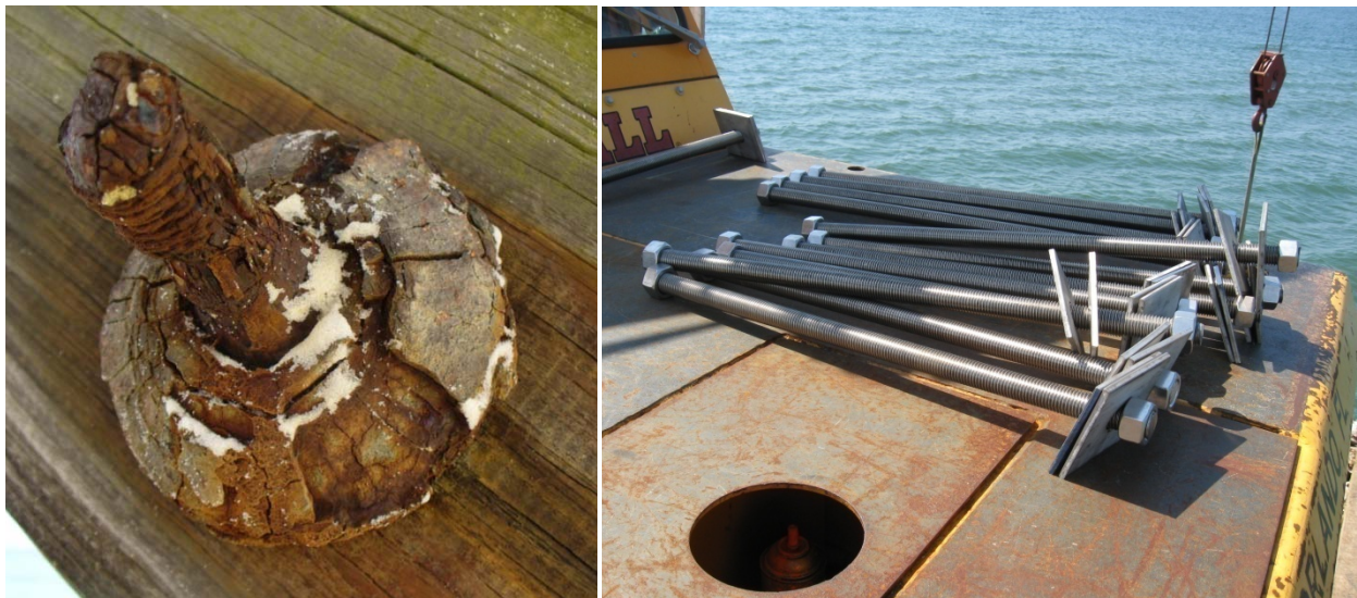
Photo 22. Corrosion of steel bolt, left; stainless steel bolts, right.
