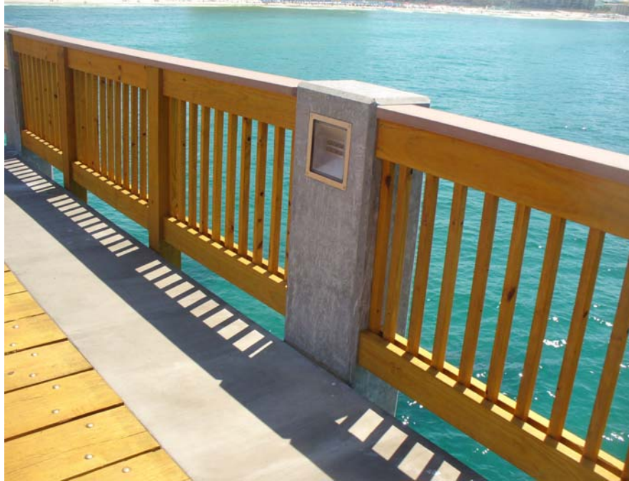
Photo 65. Concrete bollard with turtle friendly light, Russell-Fields Pier, Panama City Beach
