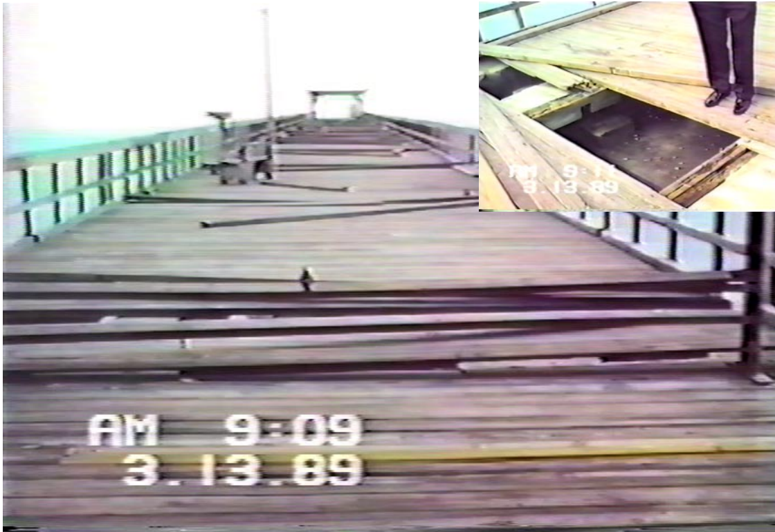
Photo 9. Selective deck damage at each bent, Lake Worth Pier [BBCS Photo Files]
