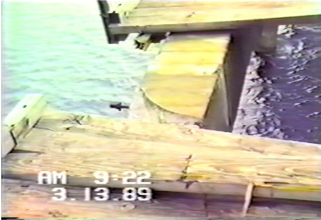
Photo 8. Pier decking damage, Lake Worth Pier (1972-2004) [BBCS Photo Files]
